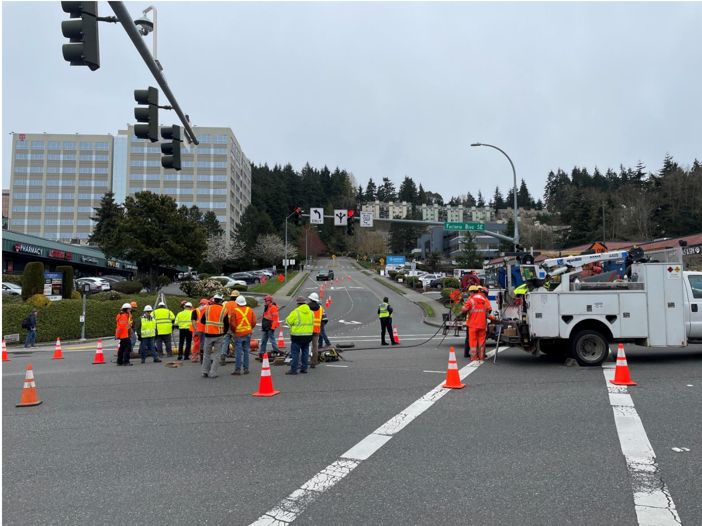
Valve that opened to 10% then froze is in the middle of the intersection in Factoria
