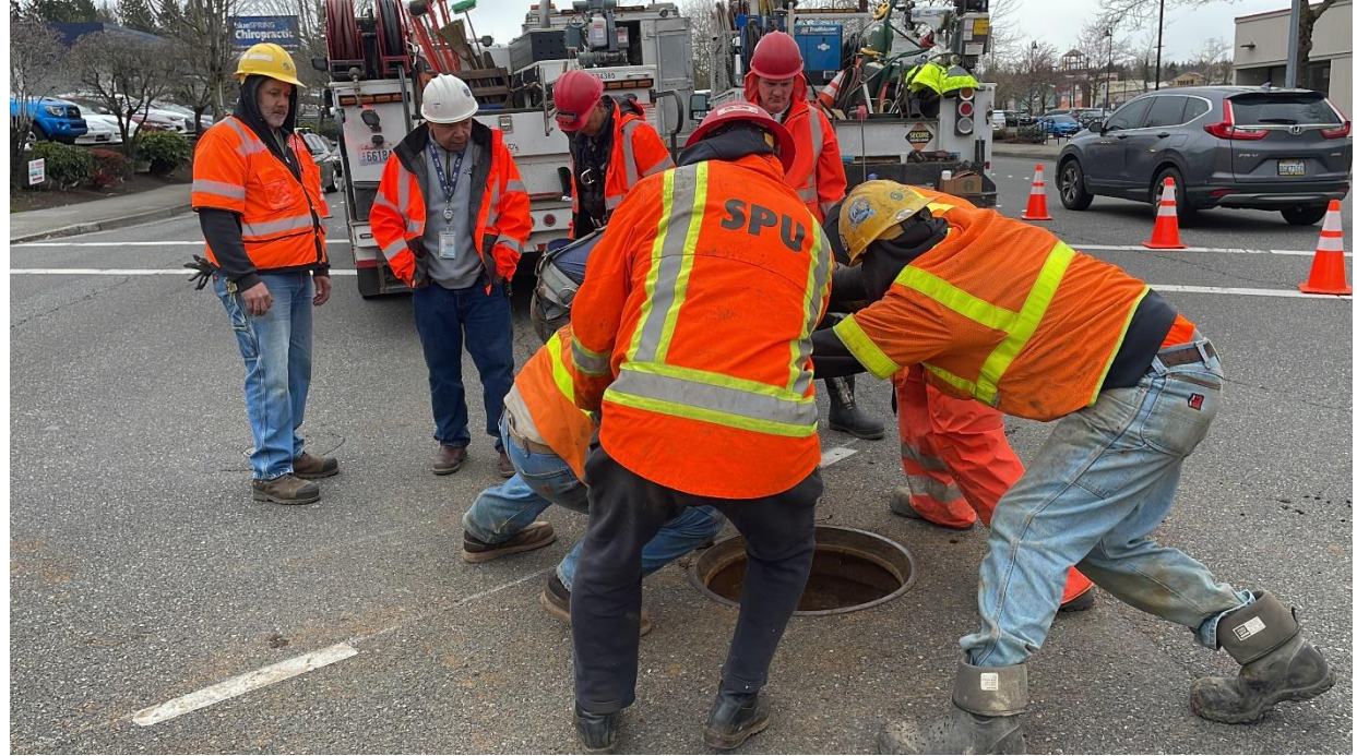
Crews manually turning the valve using a t-wrench attached to the top valve gear
