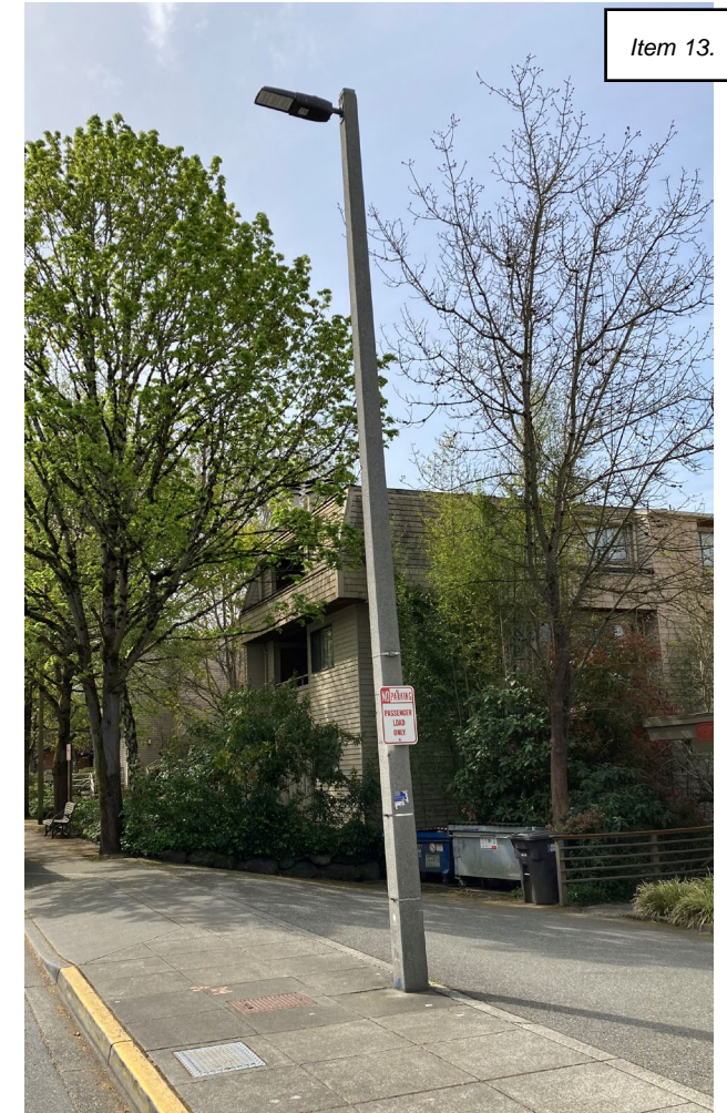
Typical concrete pole with LED light fixture
