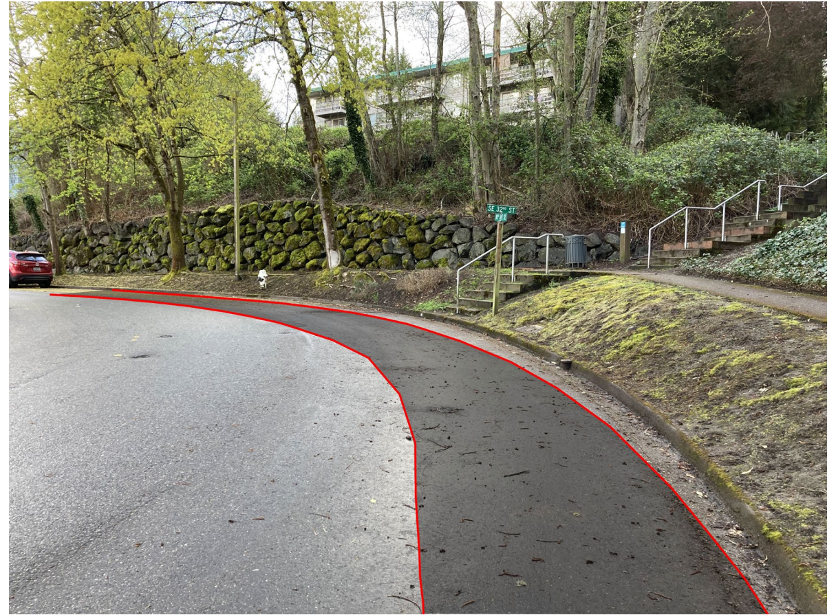
Grade difference between sidewalk and 80 th , new sidewalk to move onto street
