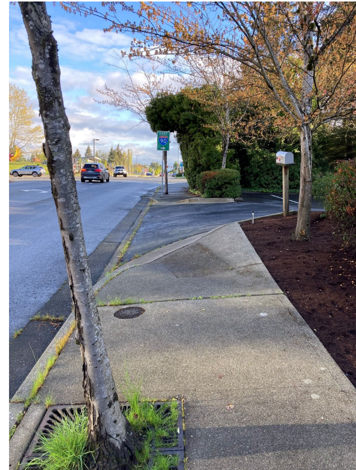
Poor ADA access at driveways
