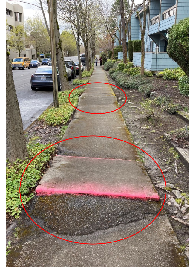
Does not meet ADA grade requirements
