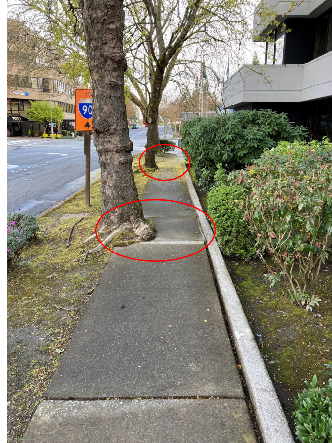
Existing sidewalk does not meet required ADA width
