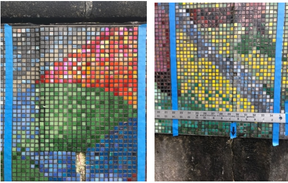
January 2024: The crack along the existing “fault line” has continued to expand causing more damage to the tilework.
