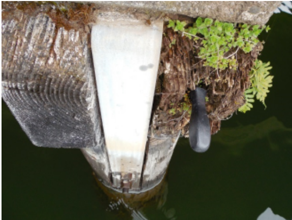
Photo 15A – Deteriorated cap beam end
