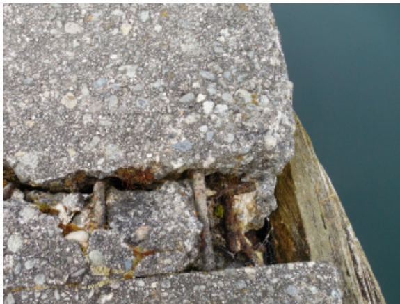
Photo 9A – Deteriorated pier slab
