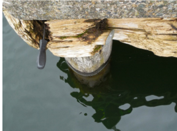
Photo 14A – Deteriorated cap beam
