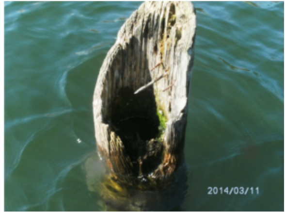
Photo 26A – Deteriorated mooring pile
