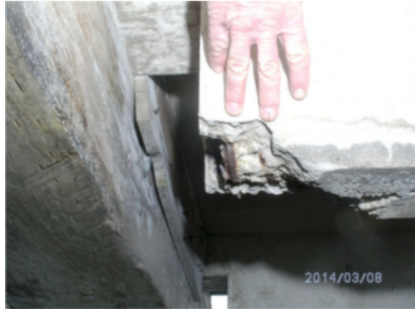
Photo 16A – Spalling at underside of precast "T"
