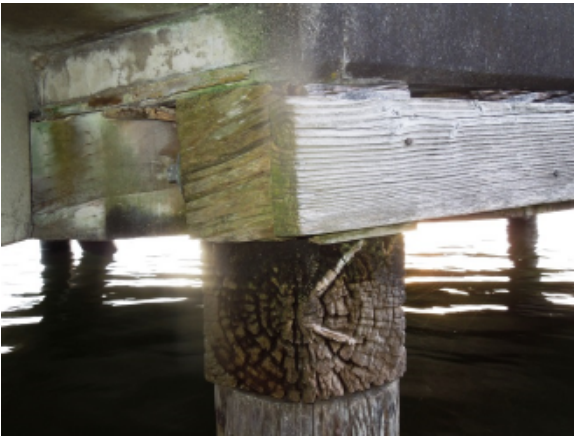
Photo 25A – Deteriorated cap beam (small pier)
