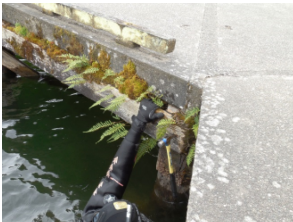
Photo 11A – Moss / vegetation at pier edge
