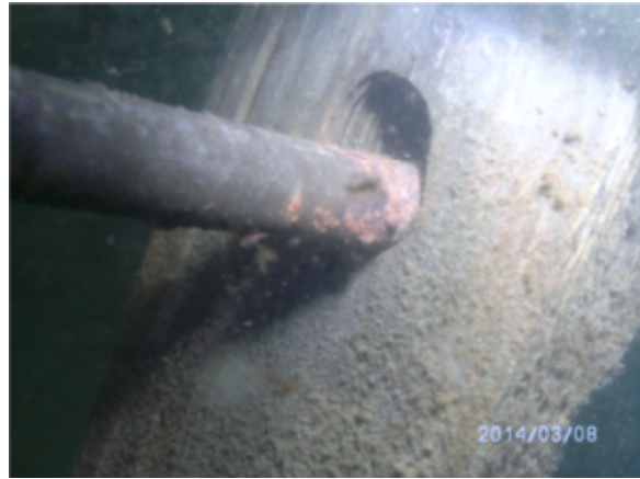
Photo 20A – Loose connector at substructure
