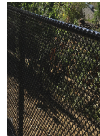
1" Coated chain link fence
