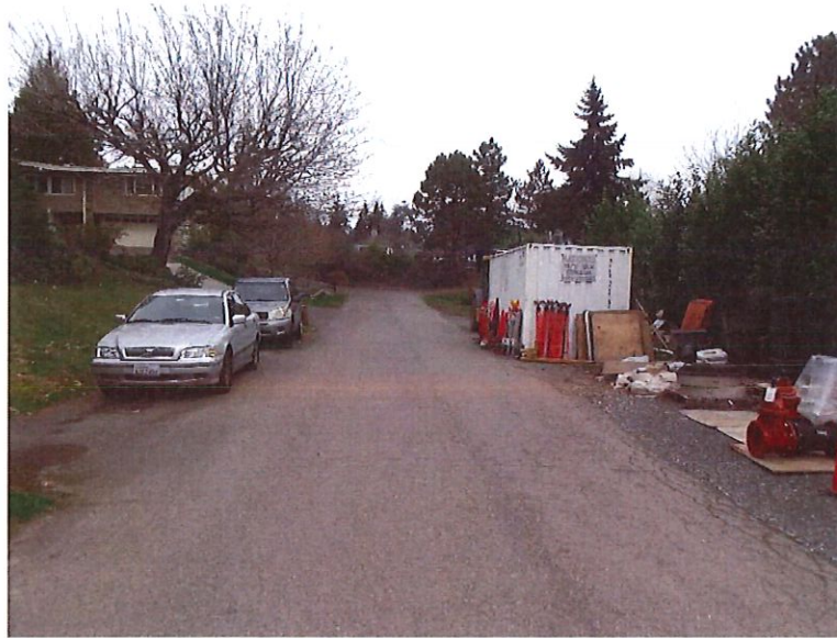
LOOKING NORTH ON 80 TH AVENUE NE WITH SUBJECT RIGHT OF WAY IN BACKGROUND SHOWING UTILITY WORK IN PROGRESS
