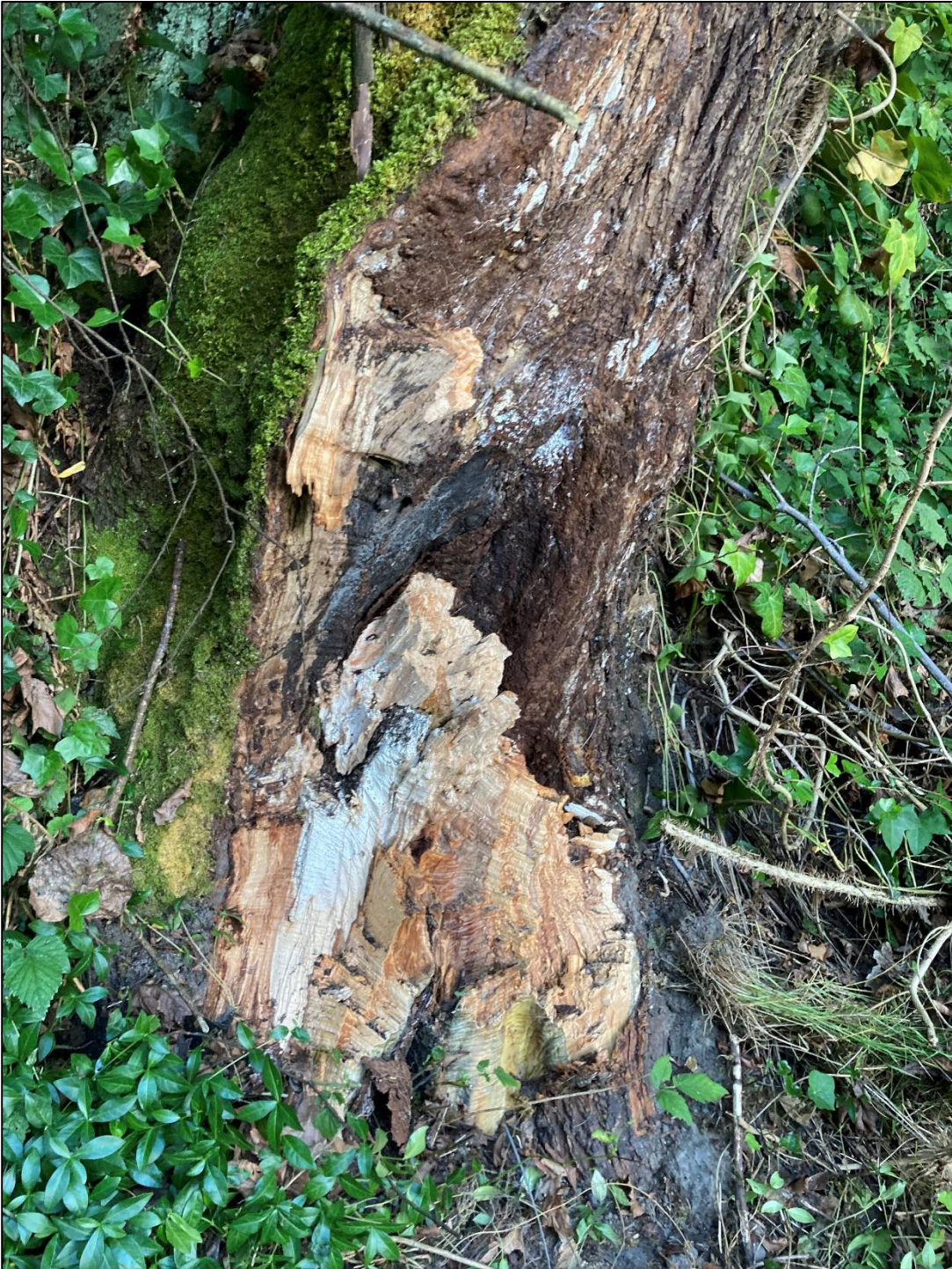
1857 Evergreen Point Road – Hazard tree assessment. Likely caused by fungal disease Kretzchmaria duesta.
