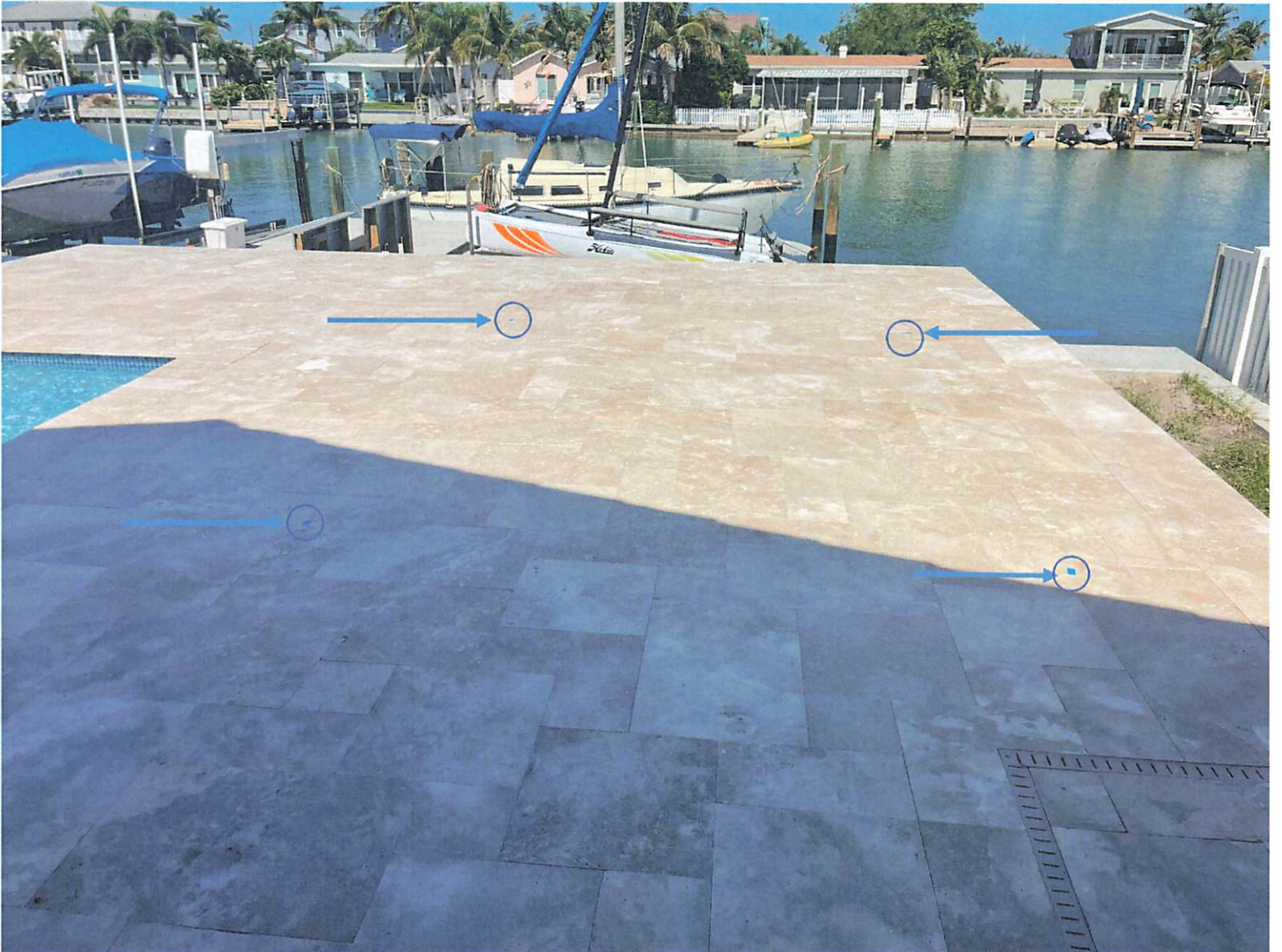
Photo of Pool Deck with Blue tape indicating location for Tiki Posts as shown on the drawing. 544 Johns Pass Ave, Madeira Beach, Fl
