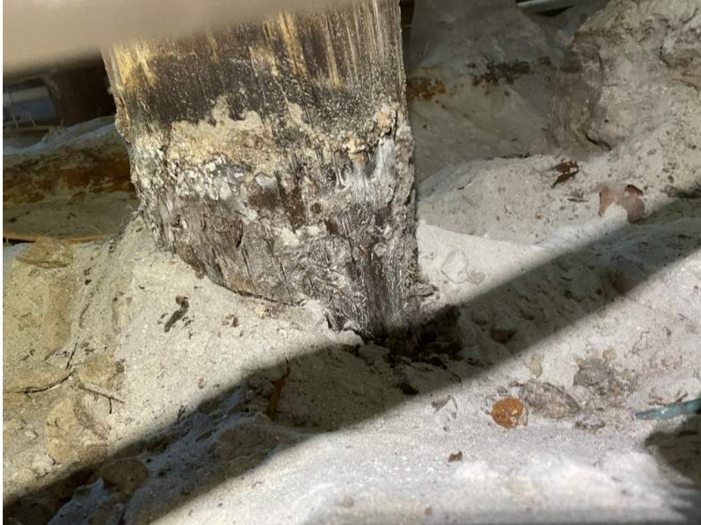
Photo 9 – Timber Pile Cross Section Loss
