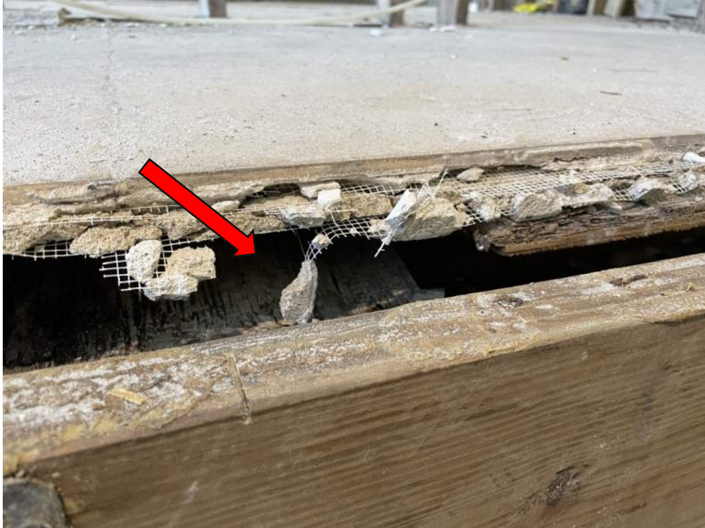
Photo 3 – Damaged or Failed Subfloor
