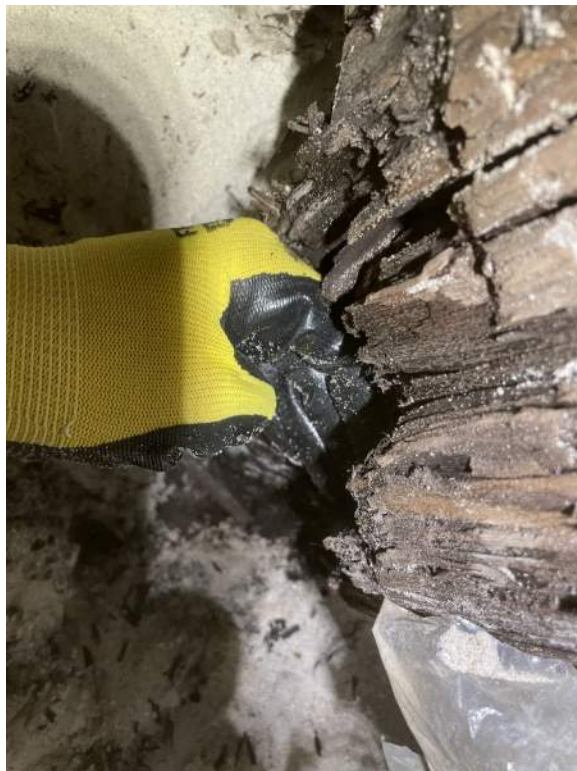
Photo 8 – Timber Pile Cross Section Loss
