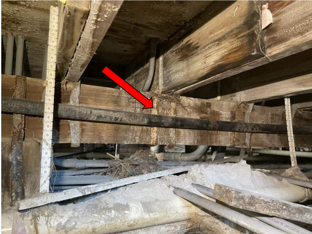
Photo 5 – Floor Joist Strap Corrosion
