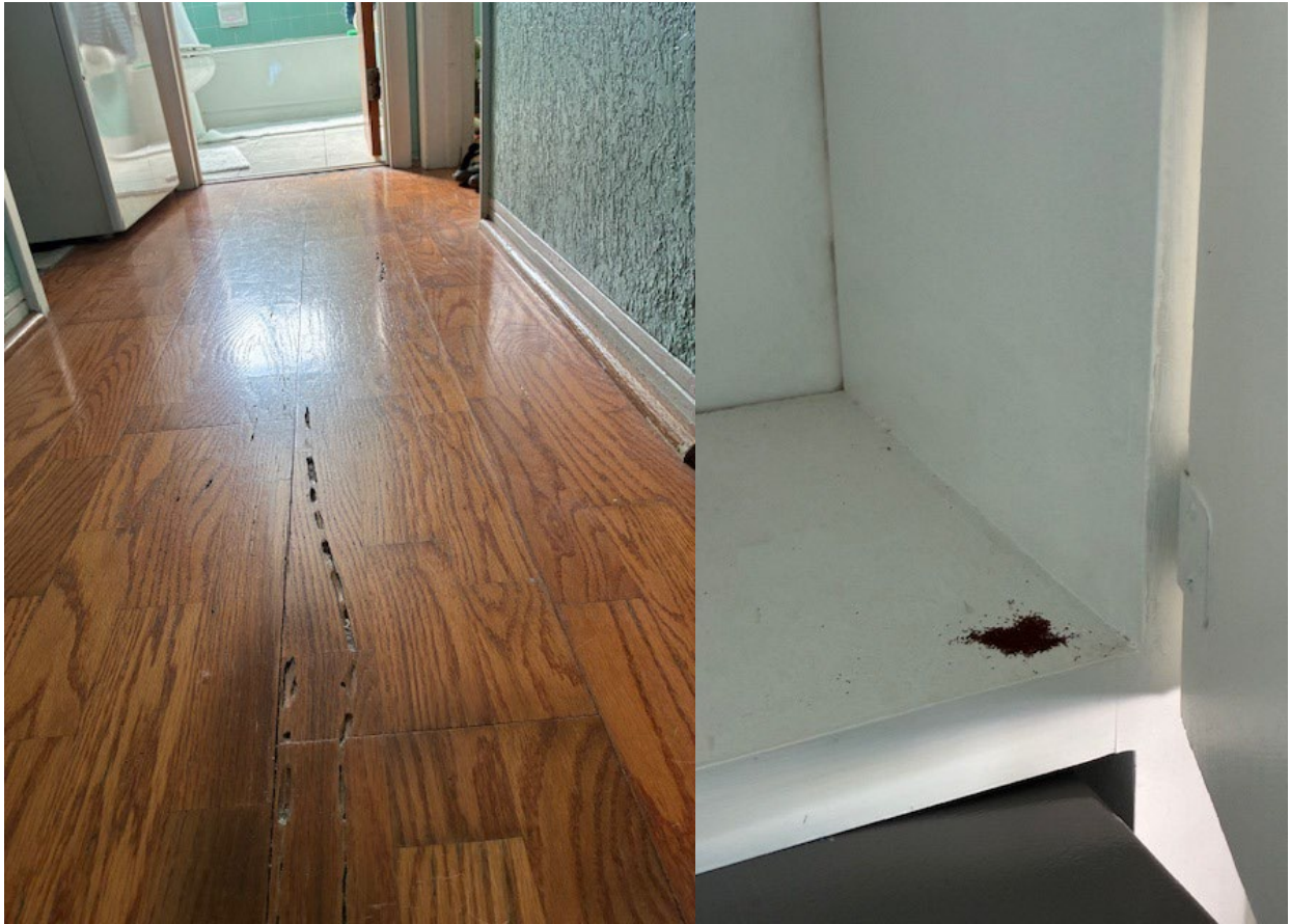
Termite damage to floor and signs of active termites
