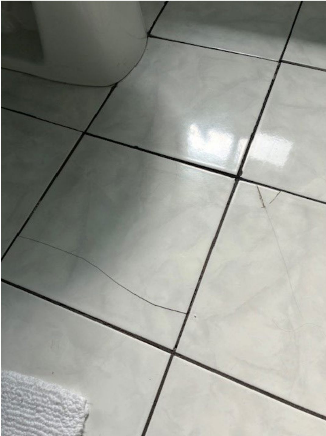
Floor/subfloor in bathroom near shower and toilet is soft and needs to be repaired. Broken floor tile needs to be replaced.
