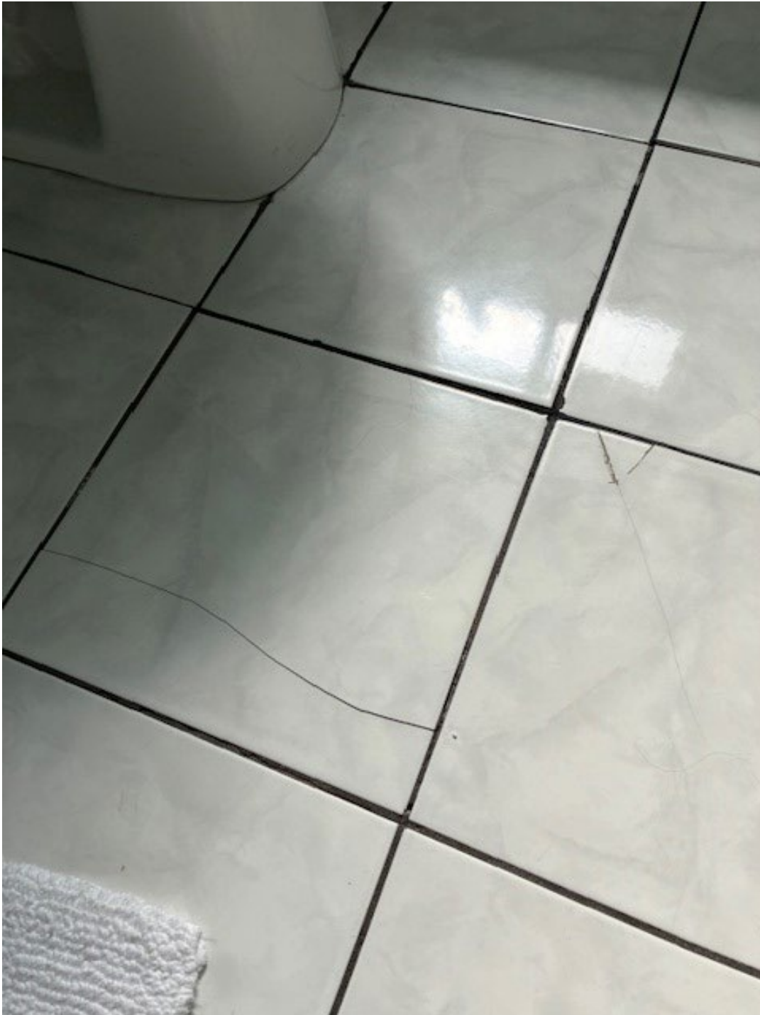
Floor/subfloor in bathroom near shower and toilet is soft and needs to be repaired. Broken floor tile needs to be replaced.
