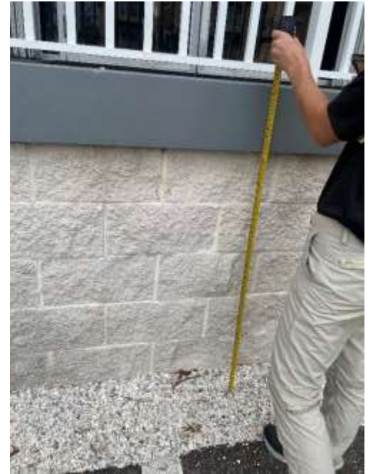
Field check – Redington Beach Town Hall is elevated mitigating some impacts shown at ground elevation.
