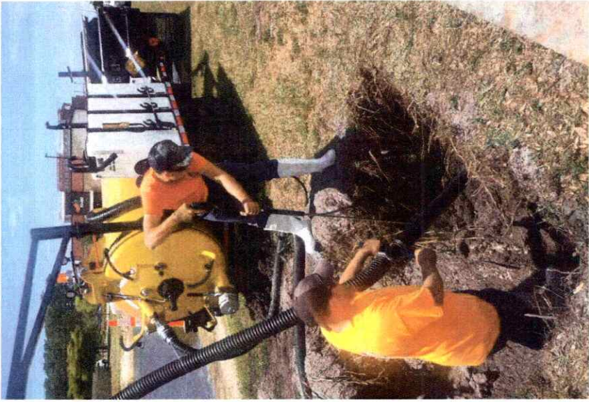
Above) An i2 Visual's team shown using their Hydro-Vac machine to dig close to utilities without damaging them. This is a very useful machine to avoid issues on today's crowded installation sites.
