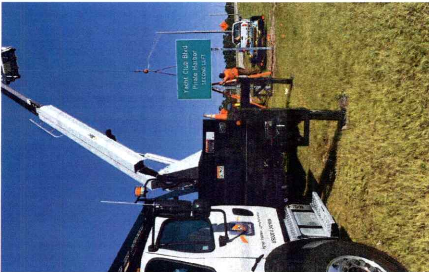
Above) One of i2 Visual's experienced install teams finishing one of two new FDOT standard multi-post traffic signs for Charlotte County Florida (footers, break-away structure and sign panel.)
