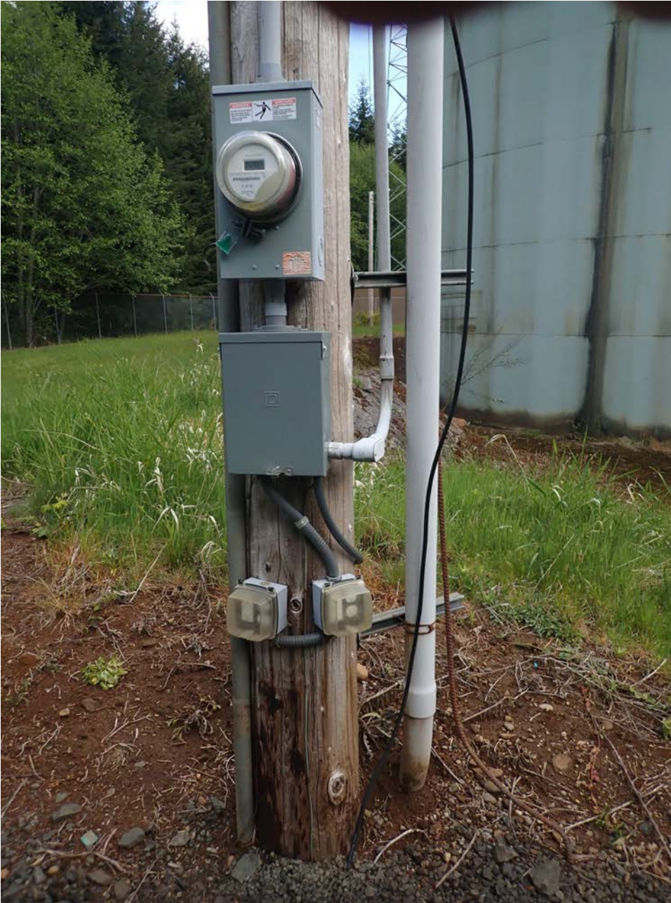
Image 9: Looking east northeast at the AC power pole that will provide power for the instrument. AC power will be converted to low voltage DC power and trenched to the post and power enclosure. The precise path of trenching will depend on the location of other buried utilities (fiber). A small repeater box will need to be mounted to the power pole to host the AC to DC power converter. An electrician will need to be onsite to pull power from the power pole.
