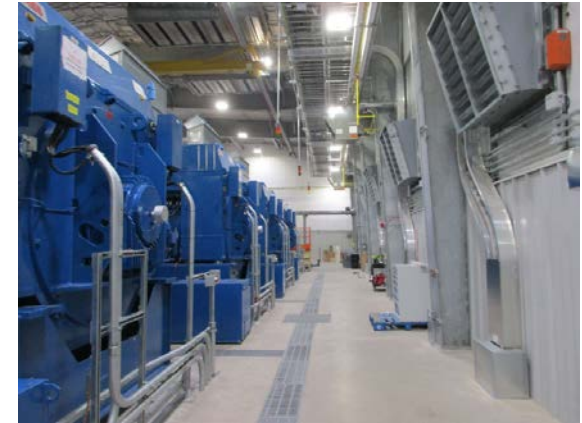
Westside Energy Station 5x9 MW
