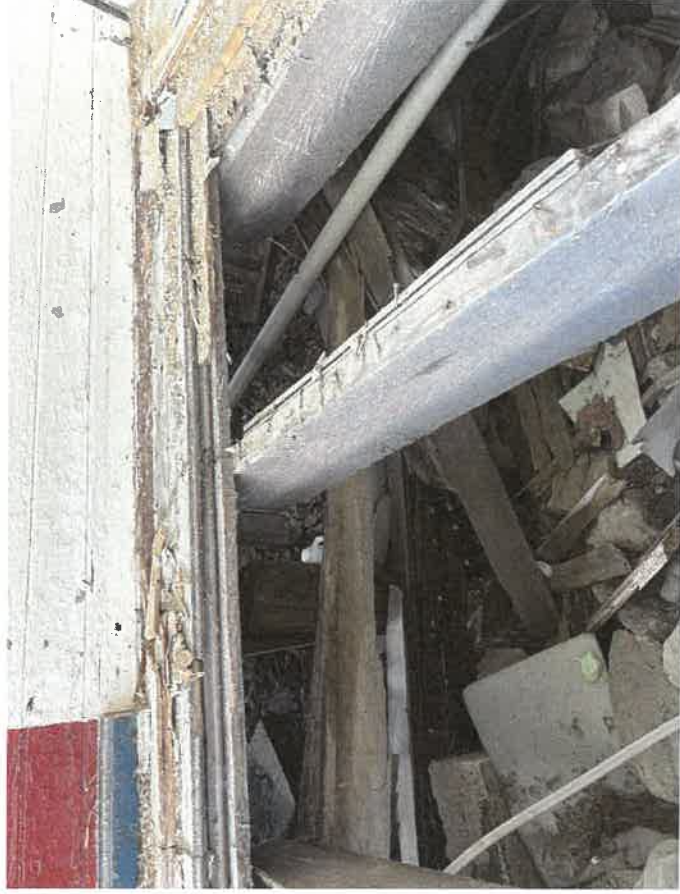
Foundation Obsolescence & Failure
