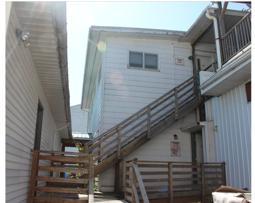
EXISTING WOODEN STRUCTURE, PORCH AND STAIR CONNECTING EXISTING SHED AND BUILDING, LOOKING WEST
