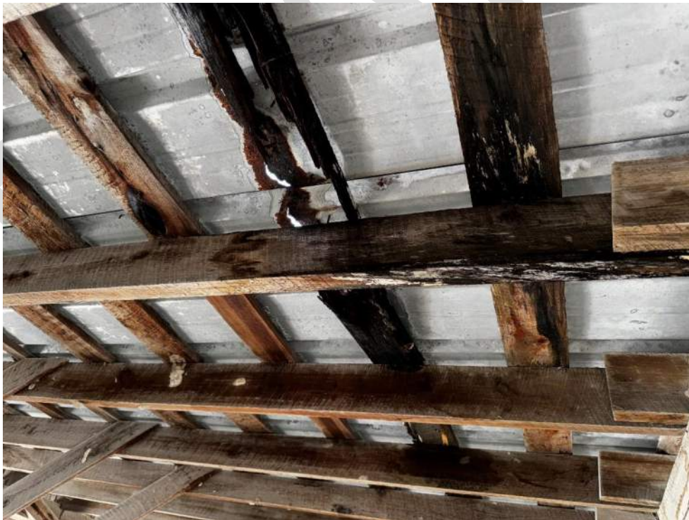
Photo 34 – View of damaged roof wood purlins, rafters, diagonal bracing and metaldeck.
