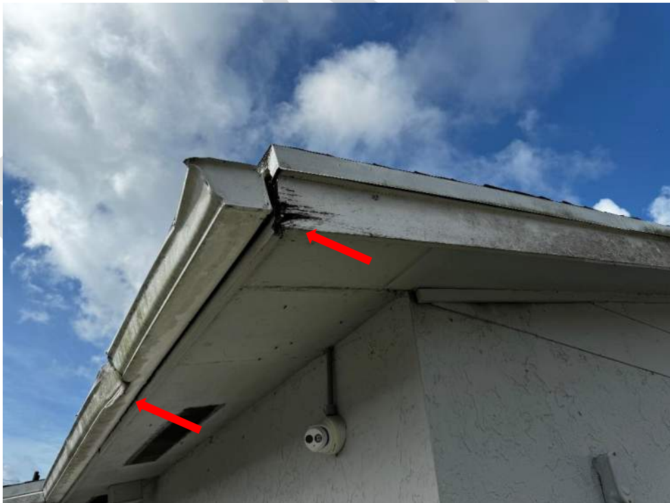
Photo 16 – View of damaged wood fascia and gutter.
