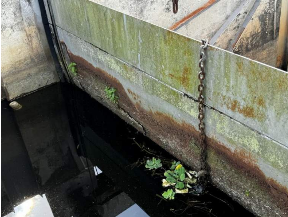
Photo 59 – View of corroded flood gate front steel plates.
