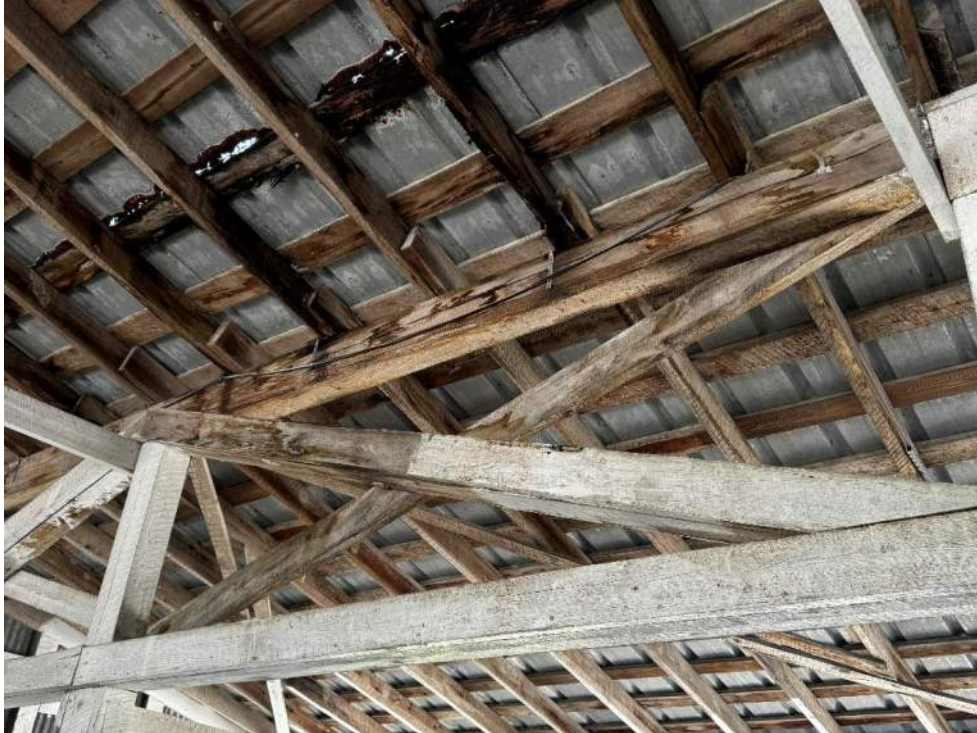
Photo 31 – View of damaged roof wood purlins, rafters, beams, cross bracing and metaldeck.
