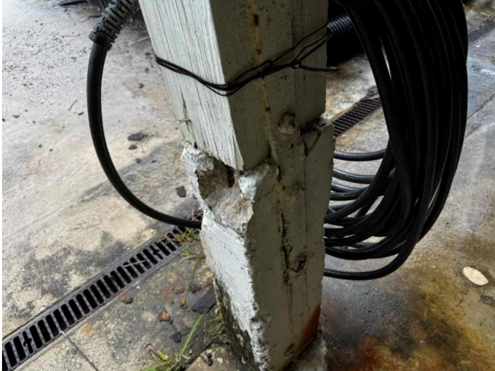
Photo 25 – View of concrete pedestal with exposed and corroded reinforcing bar. Also, corroded connector straps and bolts.
