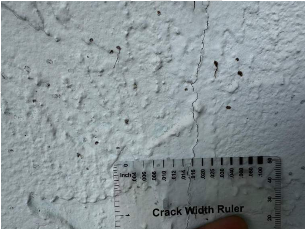
Photo 8 – View of hairline stucco cracks around the office building.
