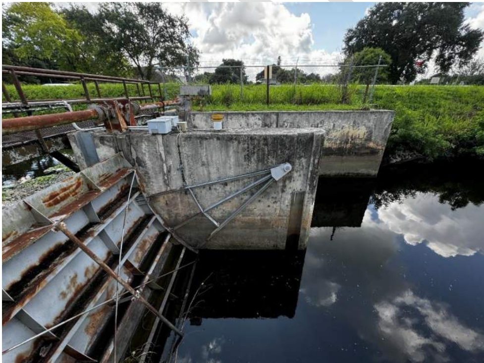
Photo 54 – View of radial flood gates, concrete wall and metal walkway at Control Structure D.
