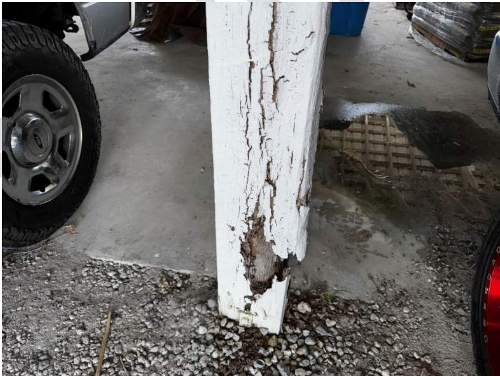
Photo 24 – View of damaged wood column with evidence of termites (Column to be shored).
