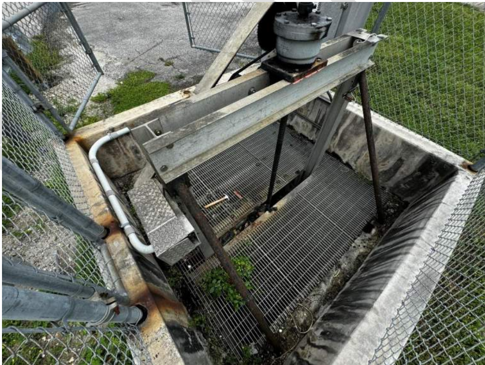
Photo 72 – View of Control Structure C slide gate support beams and diagonal bracings with light corrosion.
