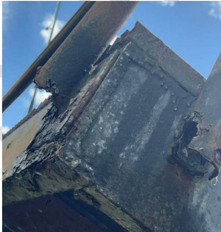
Photo 64 – View of corroded steel channels, welded guardrail posts and grating.
