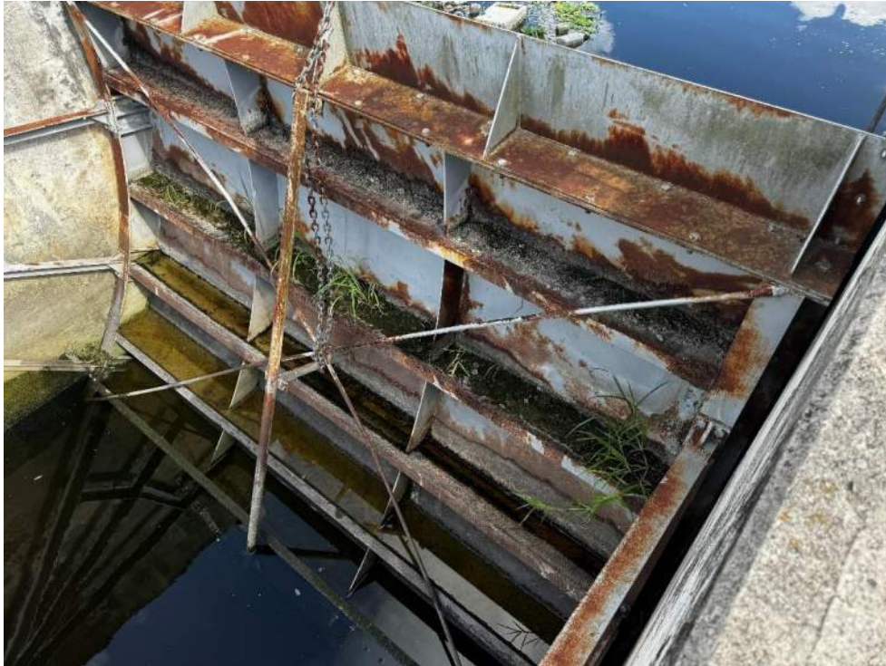
Photo 61 – View of corroded flood gate front steel plates and framing.
