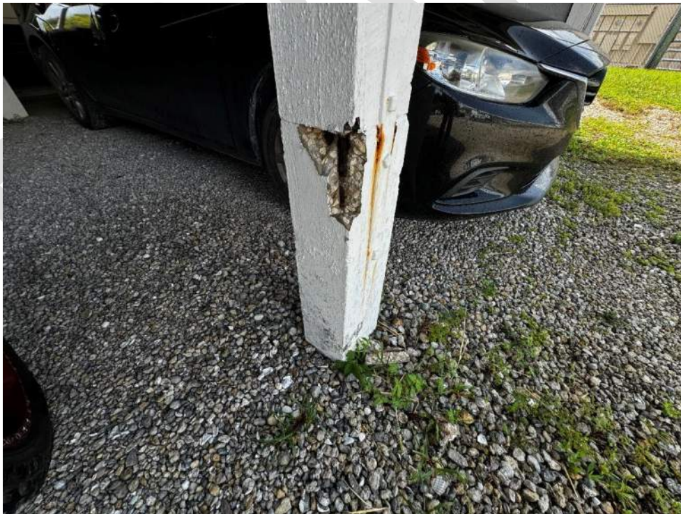
Photo 26 – View of concrete pedestal with exposed and corroded reinforcing bar.
