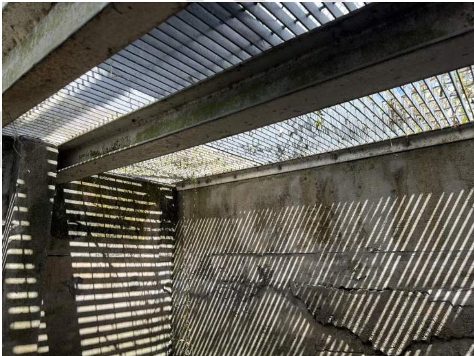
Photo 70 – View of concrete spalling on the north wall of concrete box.
