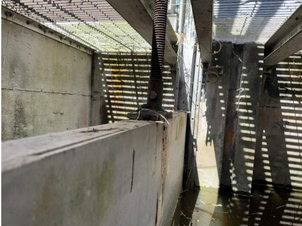
Photo 69 – View of Control Structure A interior wall and slide gate condition.
