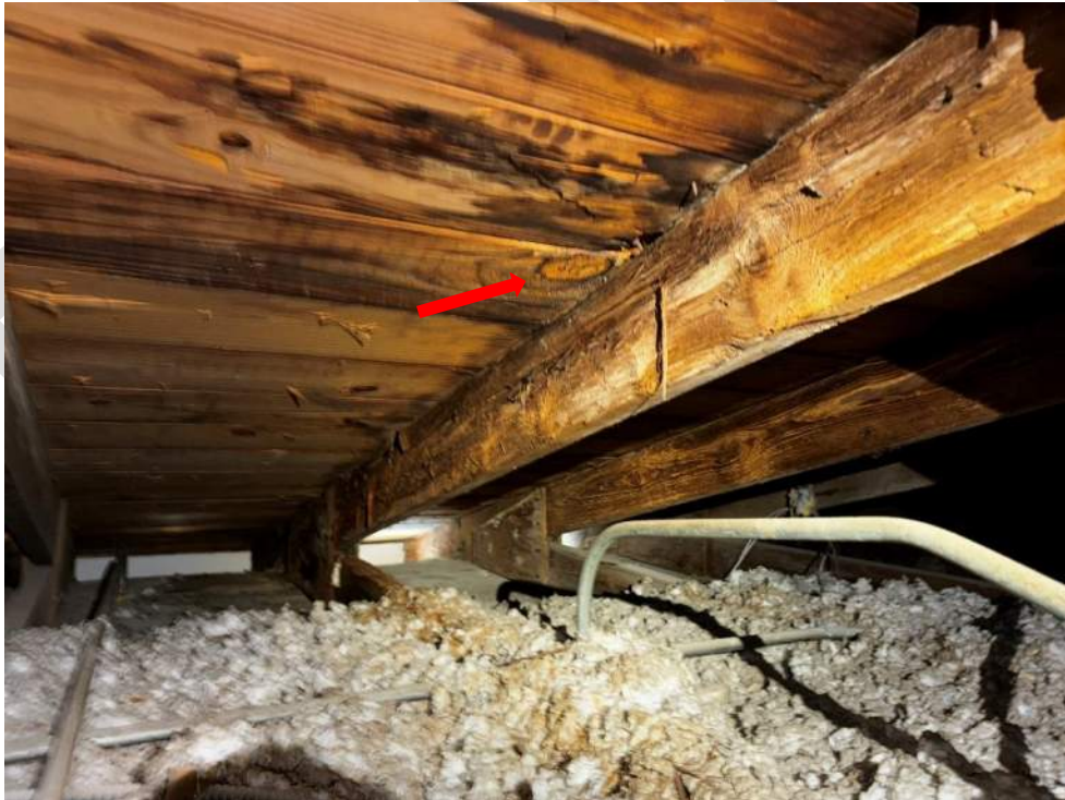
Photo 14 – View of damaged wood truss member and sheathing (From south side access hatch).
