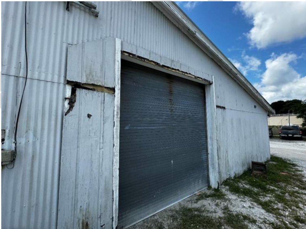
Photo 40 – View of damaged wall plywood sheathing at the north side of the wood shed building.
