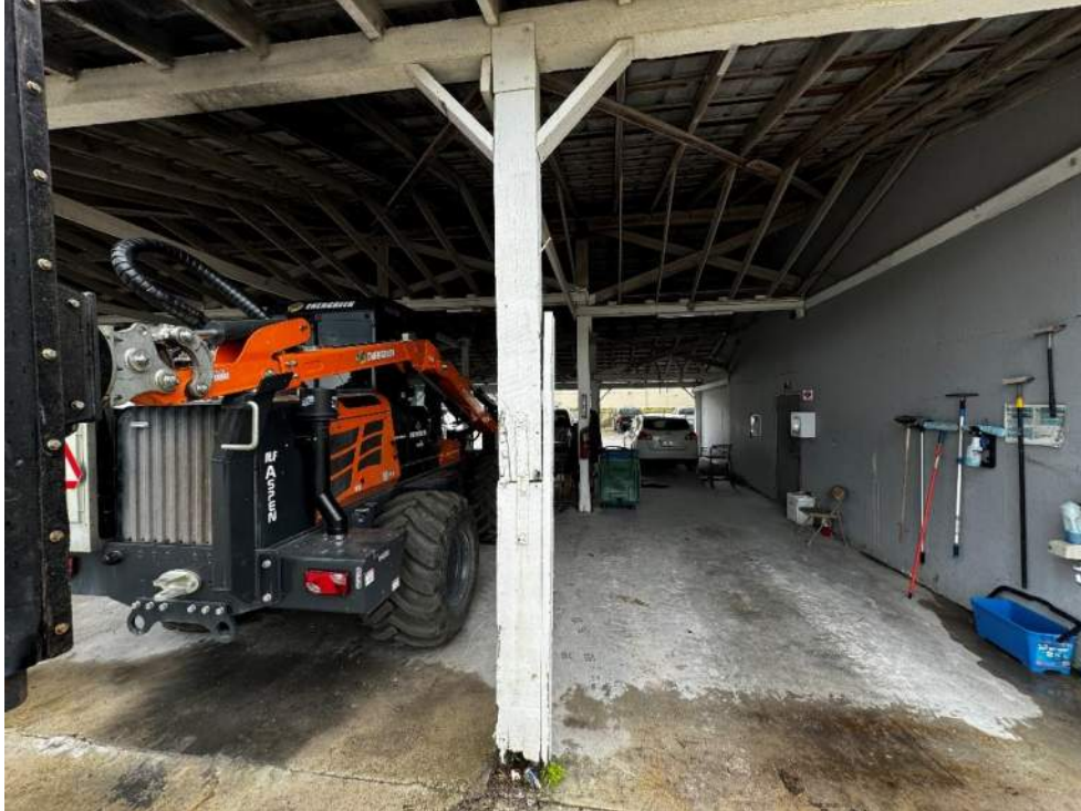
Photo 21 – View of damaged wood column with a 100% section loss (Column to be shored).
