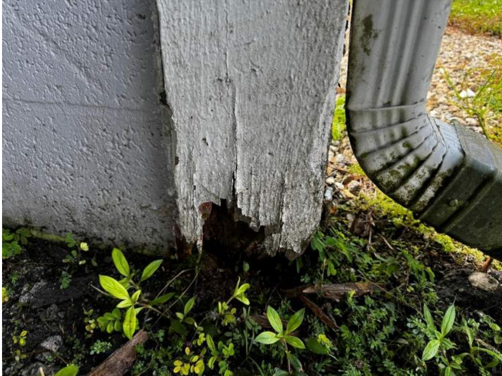
Photo 23 – View of damaged wood column at southwest corner of the building (Column to be shored).
