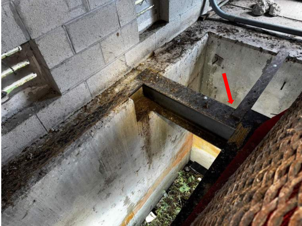
Photo 51 – View of pump-house floor steel beams condition.
