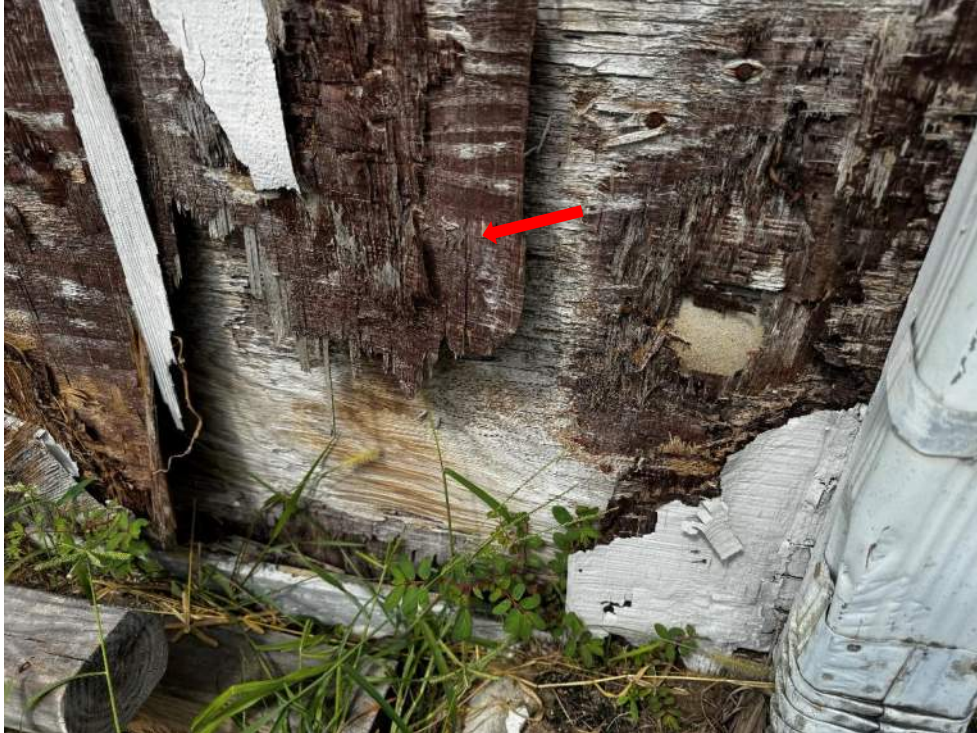
Photo 39 – View of damaged wall plywood sheathing at the north side of the wood shed building.
