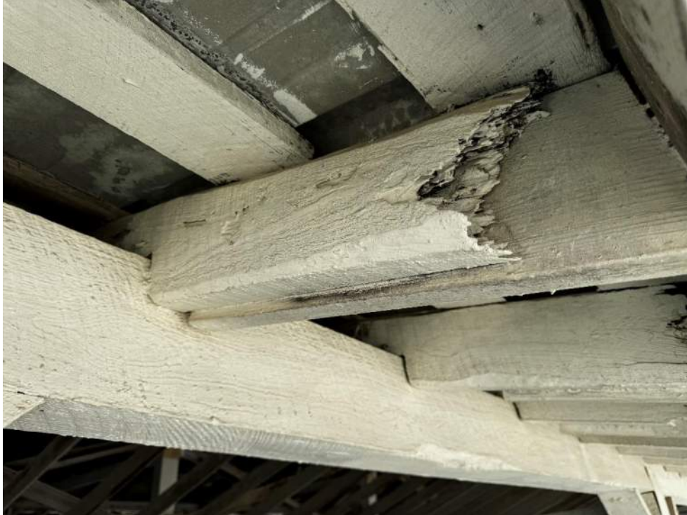
Photo 35 – View of damaged overhang rafters.
