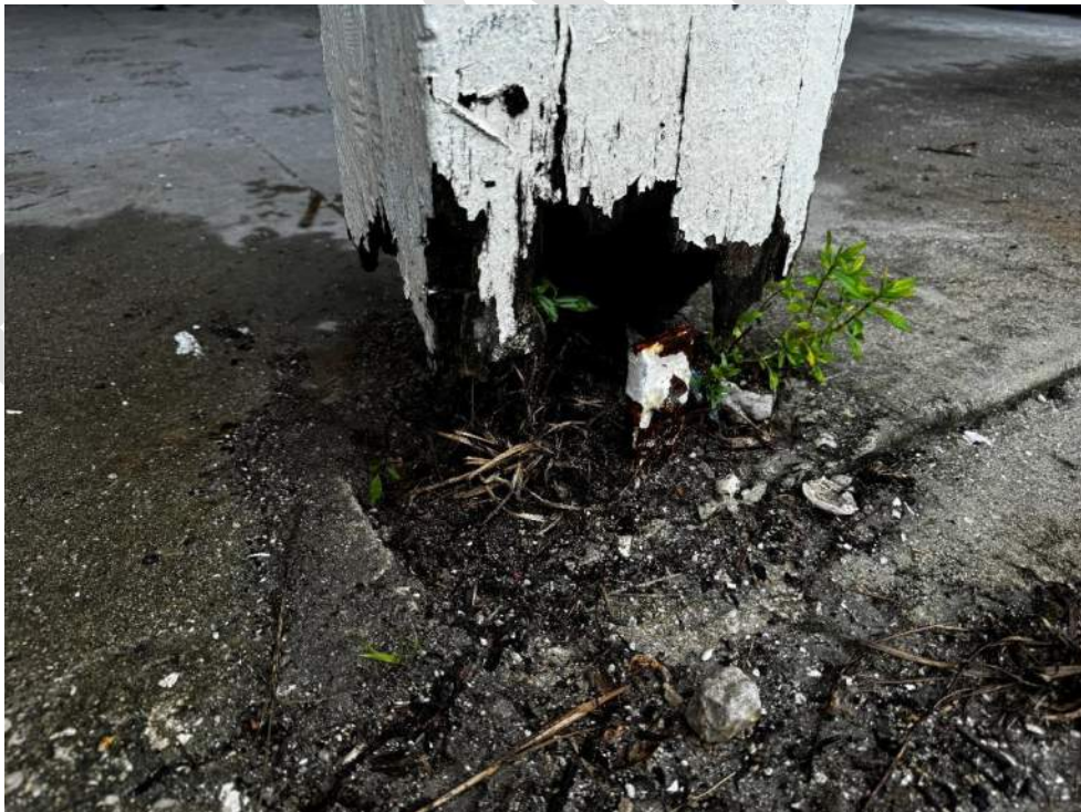
Photo 22 – View of damaged wood column with a 100% section loss (Column to be shored).
