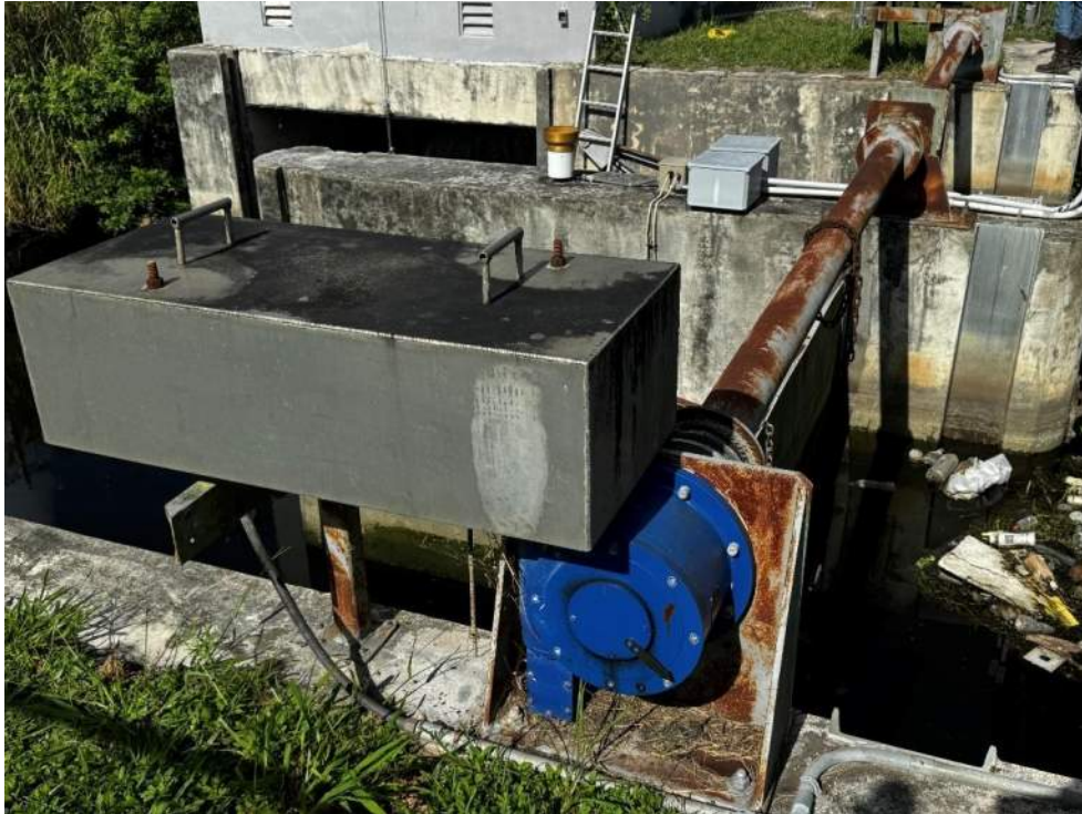
Photo 57 – View of lightly corroded radial gates hoist system.
