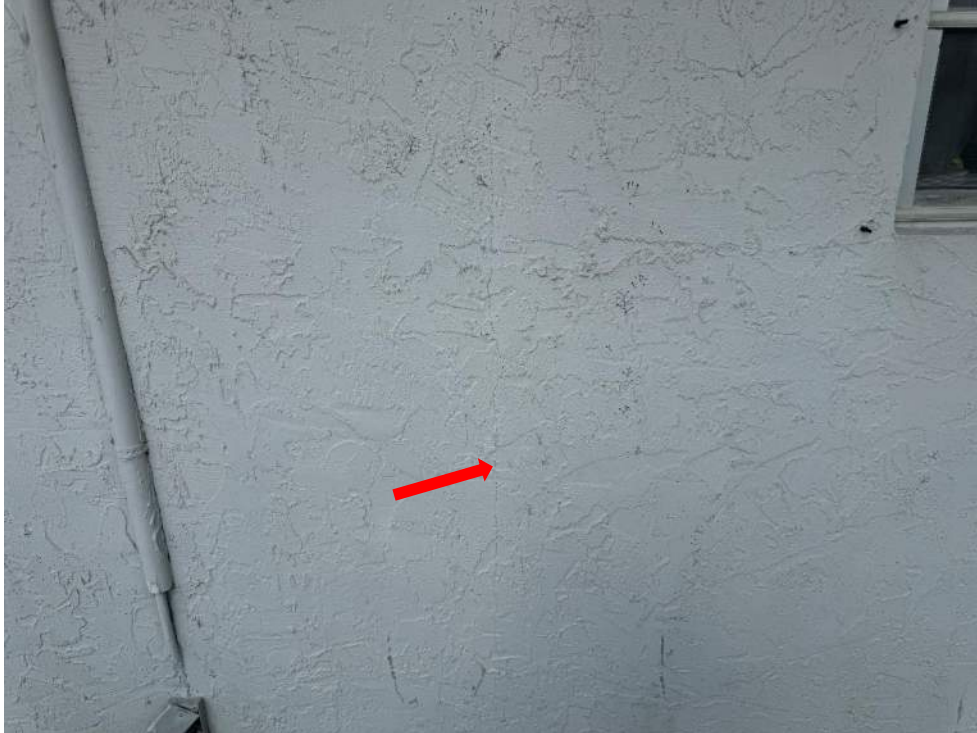
Photo 7 – View of hairline stucco cracks around the office building.
