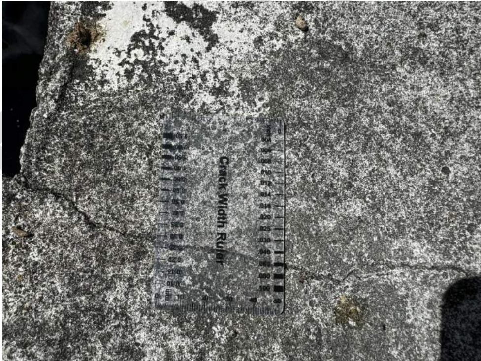
Photo 56 – View of crack at intermediate concrete pier.
