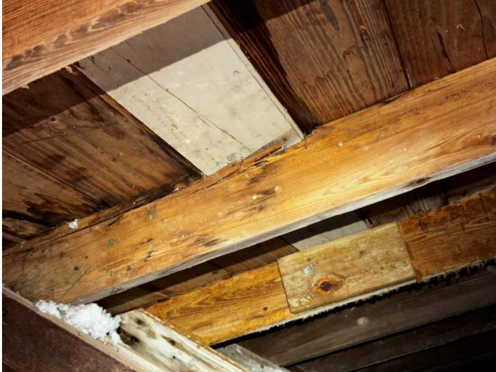
Photo 13 – View of damaged wood truss member and sheathing (From south side access hatch).
