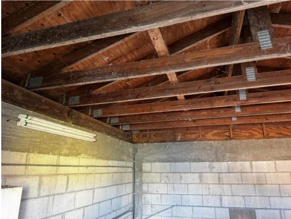
Photo 49 – View of interior condition of pump-house roof trusses, masonry wall and concrete beams.
