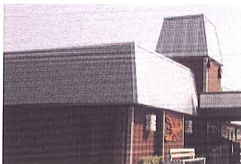
Unacceptable Hip on Deck Too Tall
