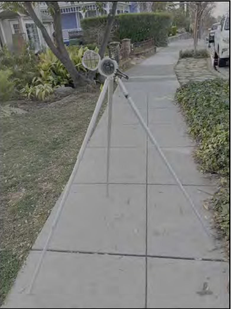
1 Place the Transit on sidewalk and sight in the maximum elevation of the roof.
