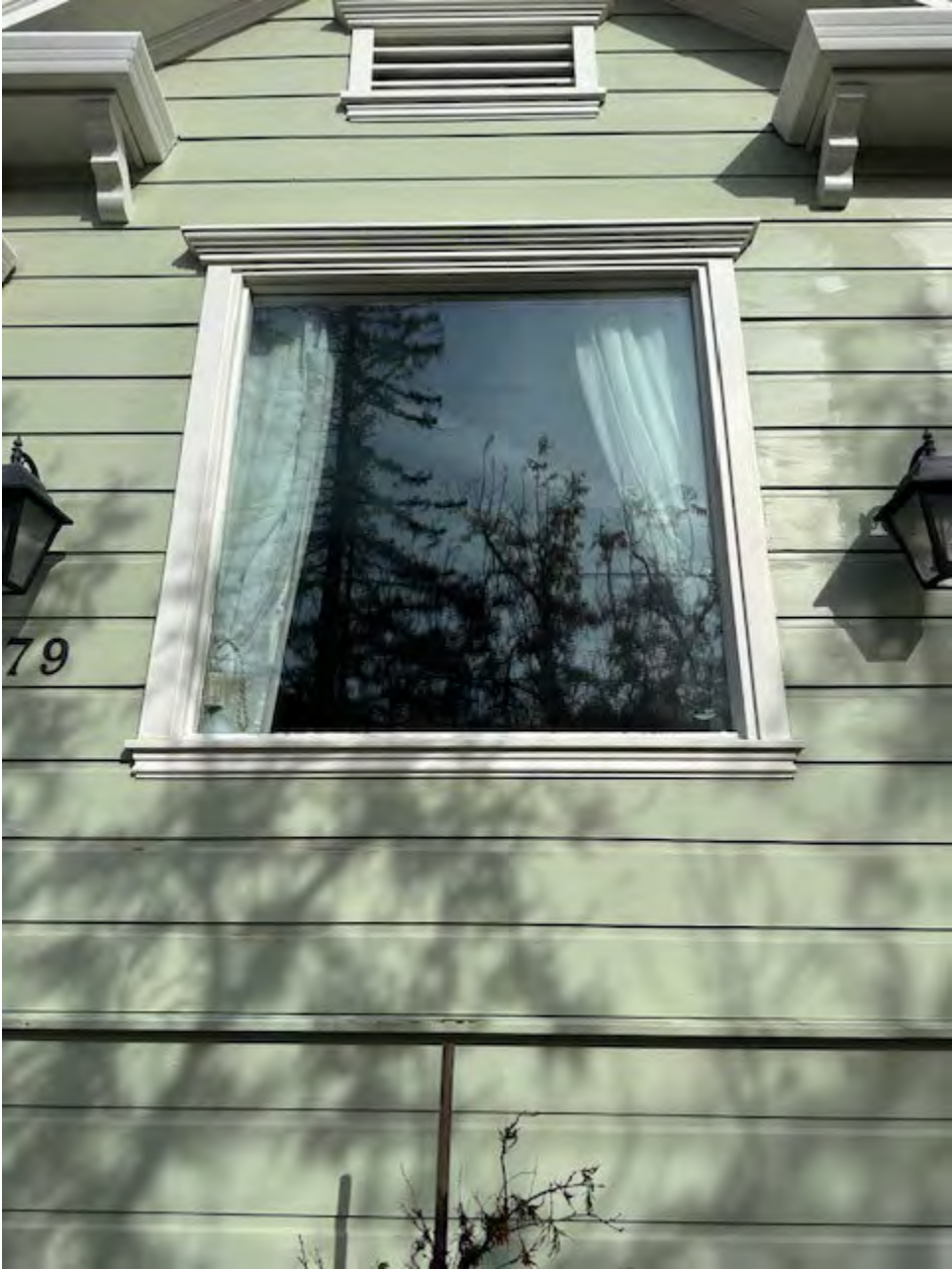
Window to be replaced
