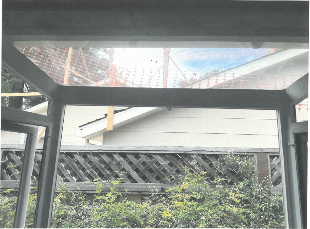
Kitchen window over sink (note: we installed this bumped-out window in our kitchen to capture more light)
