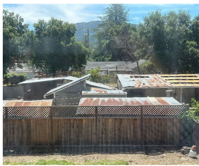
Figure 9 – View of the prior structures at 15411 National Avenue from our master bedroom (photo taken in May 2024, showing unrepaired storm damage on the roof from February 2024)
