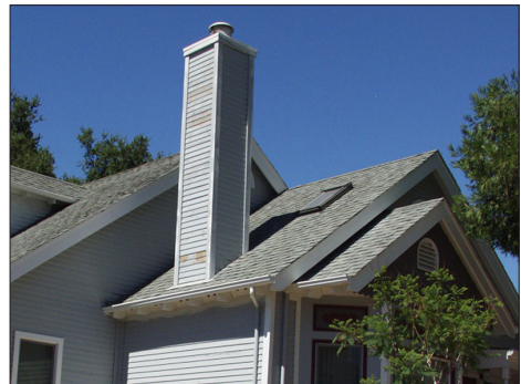
Wood clad chimneys are prohibited
