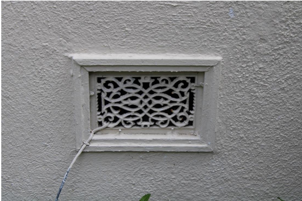
Figure 38. Cast-iron vent cover at the foundation.
