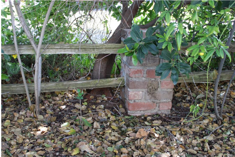
Figure 42. Fence with brick posts and wood rails along southern perimeter of the Property.
