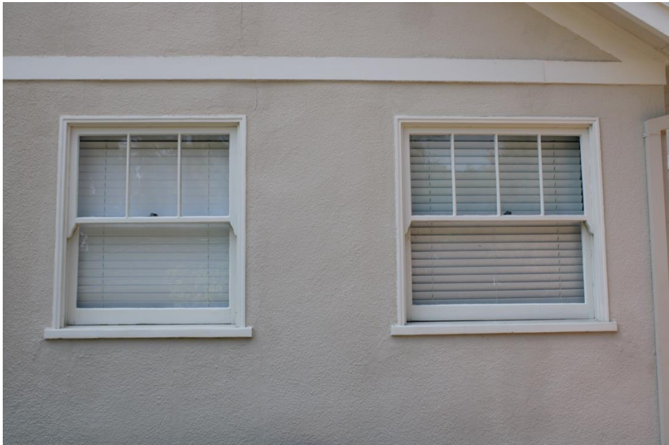
Figure 33. Three-over-one windows with horned stiles (aka lugs) on the east elevation, facing west.
