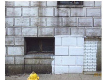
[1] A test patch should always be done before using a chemical cleaner to ensure that it will not damage historic masonry, as in this instance, terra cotta.
