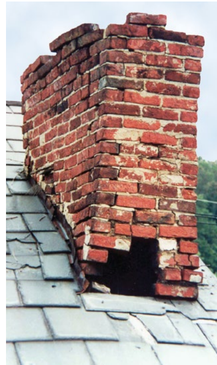
[7 a-b] This crumbling chimney was restored to its historic appearance using matching bricks.
