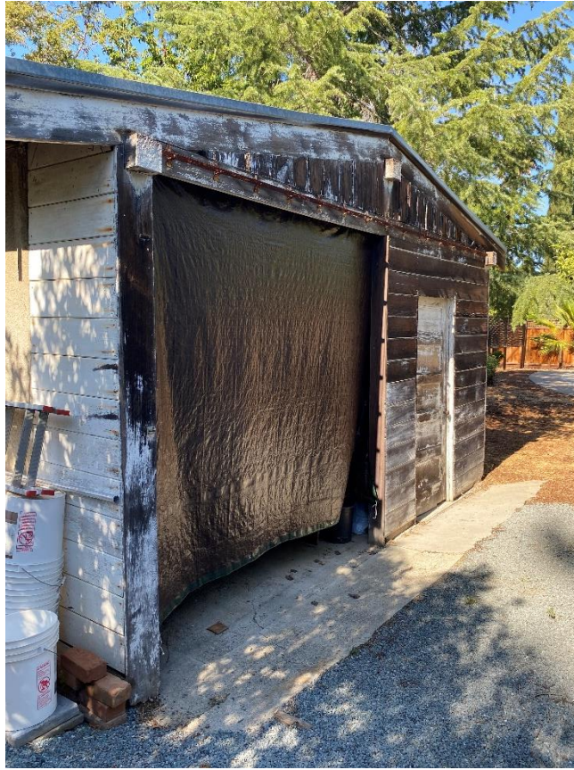
Figure 34. Photograph showing the tarp covering the wide door opening and the front entrance to the shed.
