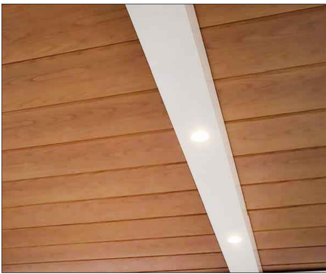
PERGOLA RECESSED DOWN LIGHTS
