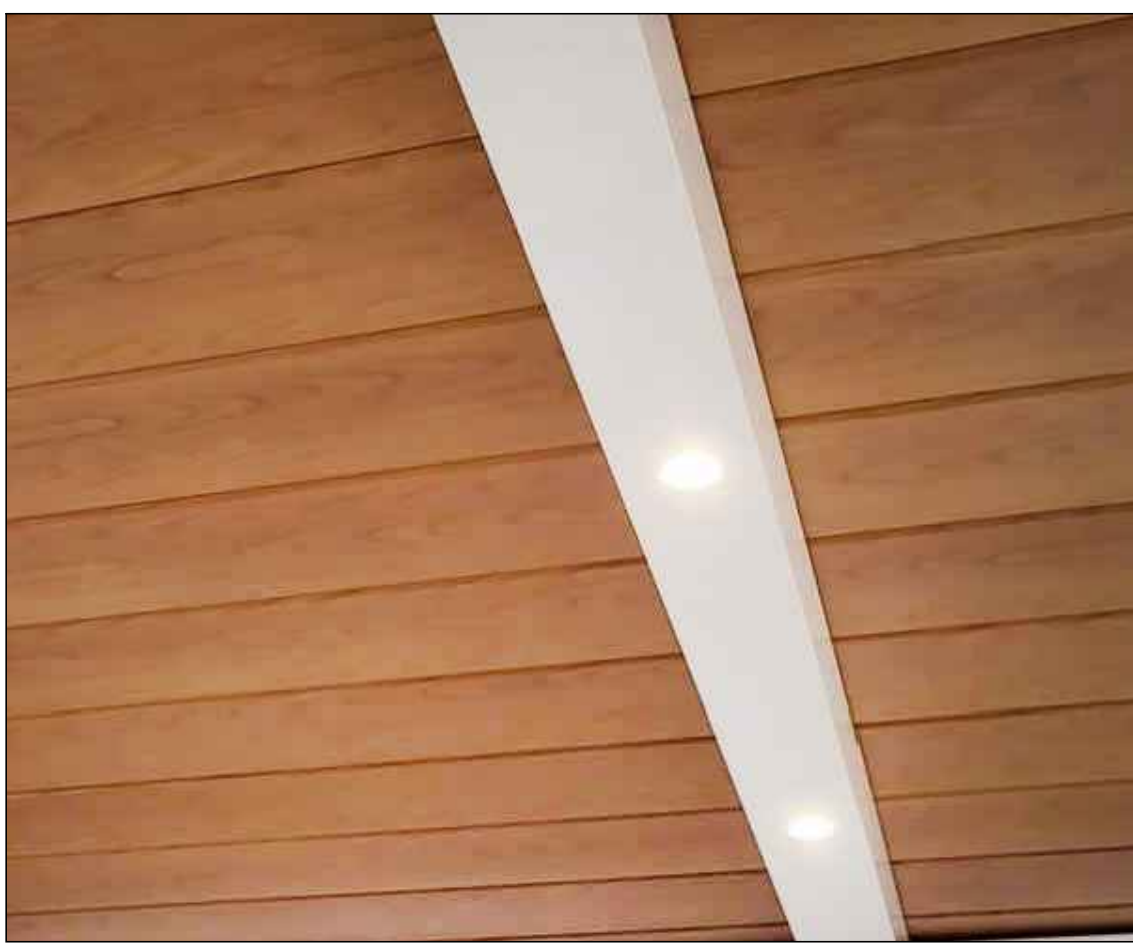
PERGOLA RECESSED DOWN LIGHTS
