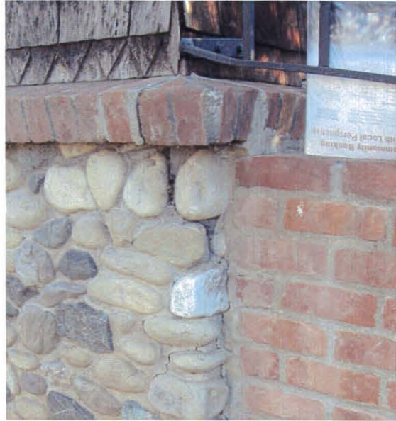
Cracks in the stone masonry will remain, but failing mortar in the brick masonry (a very limited amount) and gray Portland cement based mortar may be removed (without damaging the brick) and the brick may be repointed with a mortar that will be softer than the existing and match the existing in color.
