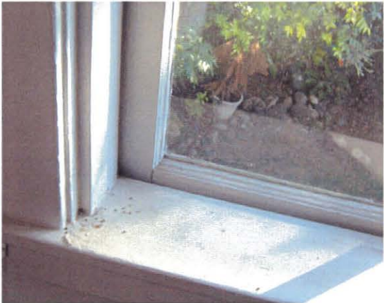
Image showing warped casement sash in the western grouping of casement windows at this elevation.
