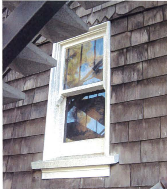
This is one of four windows proposed for removal from the first floor during phase 1. (The other three windows are at the north elevation: they are proposed to be replaced with doors.) This window illuminates the laundry room and is largely concealed behind the exterior staircase.
