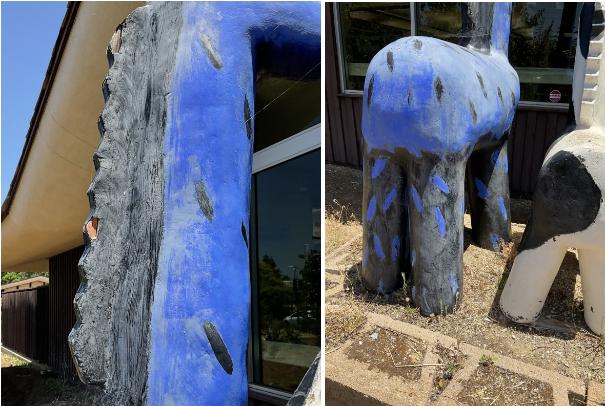
Detail of Losses Exposing Underlying Wood
