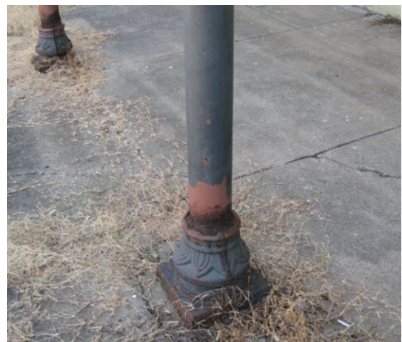
[7] (a) After the damaged portions of the base were repaired, (b) the cast-iron columns were cleaned and repainted to protect the metal from rusting.
