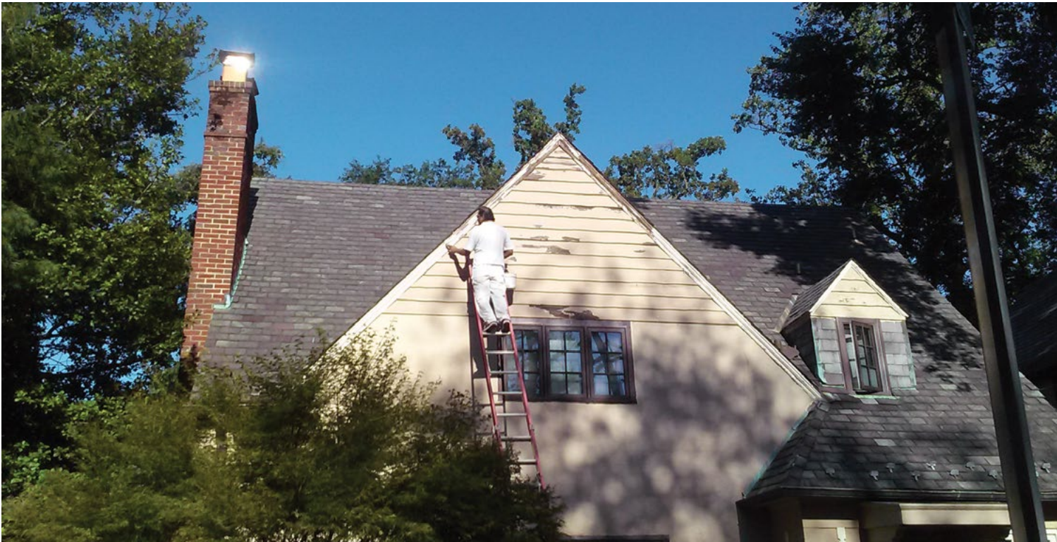
[4] Hand scraping to remove peeling paint from wood siding in preparation for repainting is an important part of regularly-scheduled maintenance.
