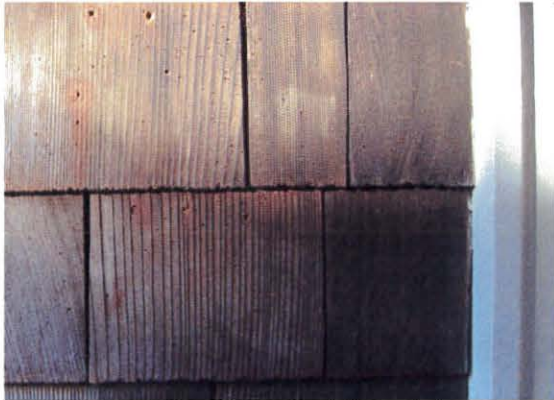
Detail view of north porch shingles which appear to be sawn redwood. These shingles are probably original to the building.
