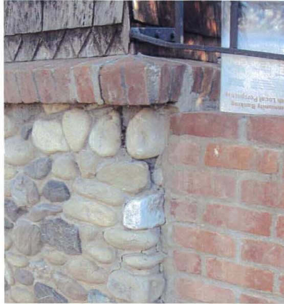
Cracks in the stone masonry will remain, but failing mortar in the brick masonry (a very limited amount) and gray Portland cement based mortar may be removed (without damaging the brick) and the brick may be repointed with a mortar that will be softer than the existing and match the existing in color.
