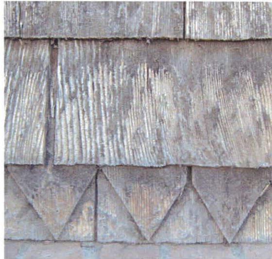
View of wood shingle deterioration due to the loss of lignin, probably caused by ultra-violet light.
