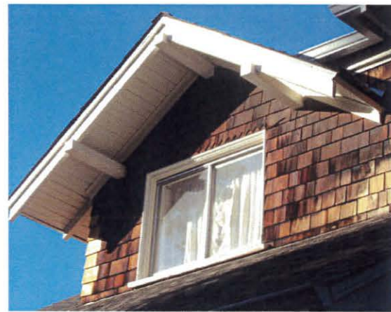
View of the easternmost windows at the second floor. These windows are not original nor are they considered historic. The windows will be replaced with double glazed wood casement sash with applied exterior and interior grids to suggest four lights per leaf. Please see window cut sheets incorporated into the drawings. The drawings show a new window to the right of the above window; it will be similar to the new sash proposed for the above opening, but double hung.
