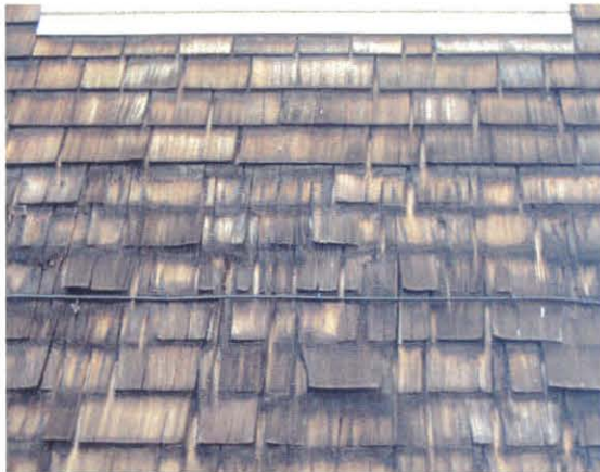
View of wood shingle damage at the south side of the west wall, between the first and second story windows. Damaged shingles will be replaced with cedar shingles. Less than 10% of the shingles need replacement. Transparent shingles stains will be tested to determine if staining will blend the new with the old; if successful, the new shingles will be stained to blend new shingles with the adjacent old shingles.
