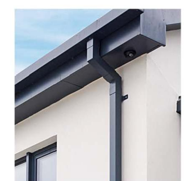
GUTTERS / RWLs Extruded Aluminum gutters Rectangular Rain Water Leaders Color: White / to match paint
