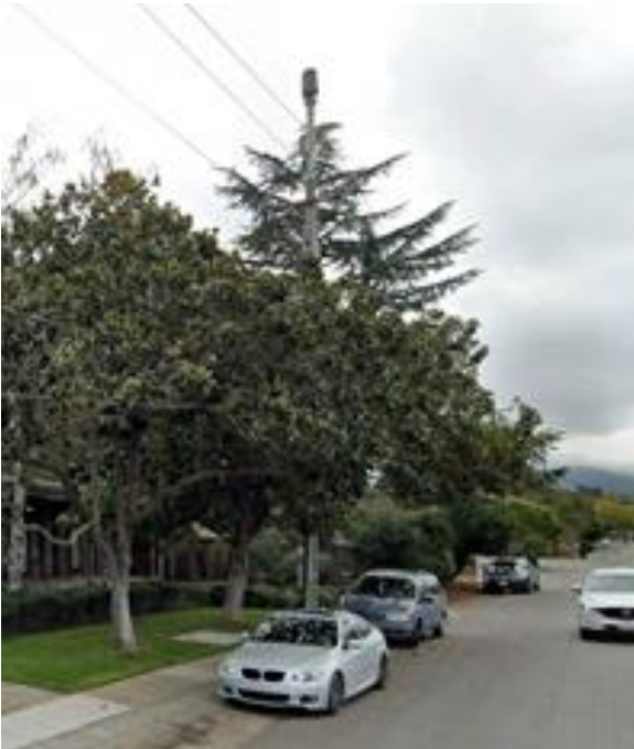
Figure 7: Landscaping conceals wireless telecommunications equipment mounted on the exterior of this pole located on Distel Drive.
