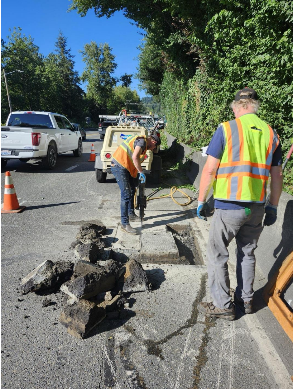
If you need a catch basin raised, we've got you covered. Our Public Works crews worked on this catch basin on Bothell Way adjusting it to ensure water flows off the street as it's supposed to.
