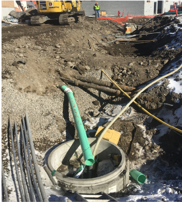
The crew is working on new manhole 103 and exposed existing power, gas and process drain line.
