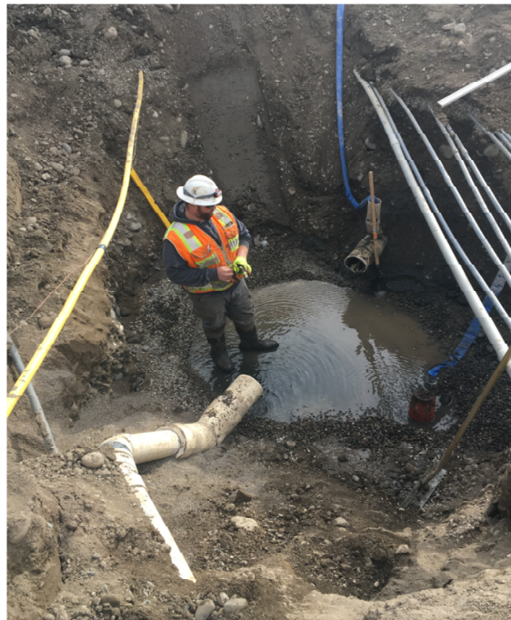
The crew is working on a new manhole installation around various existing utility lines.
