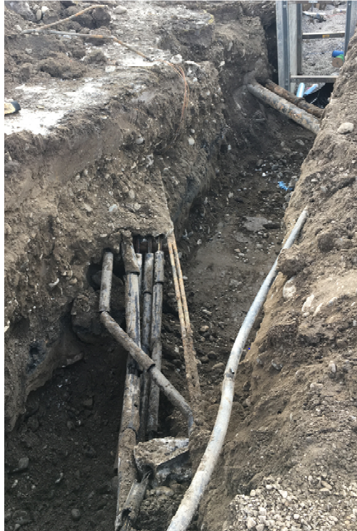
Influent line trench. An old power line (not in service) found along with some process piping.
