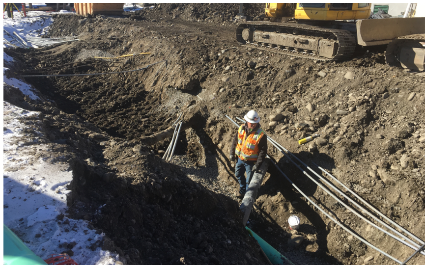
The crew is working on new sewer line and exposed multiple electric Conduits along with existing gas and process piping.
