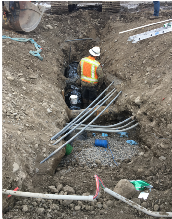
The crew is working on the new influent line around the existing electric and process piping.
