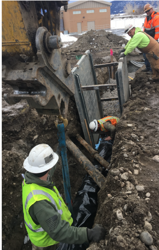
The crew is working on influent line and exposed the existing process piping.
