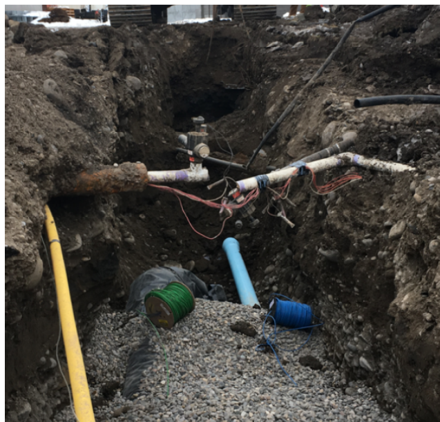
The crew is working on the re-claimed water line and exposed existing gas, process and irrigation line.
