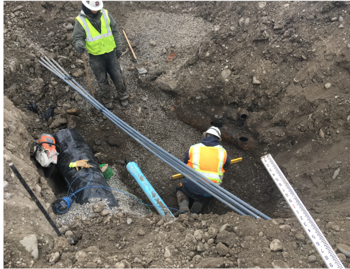
The crew is working on the new influent and re-claimed piping around the existing electric conduits.
