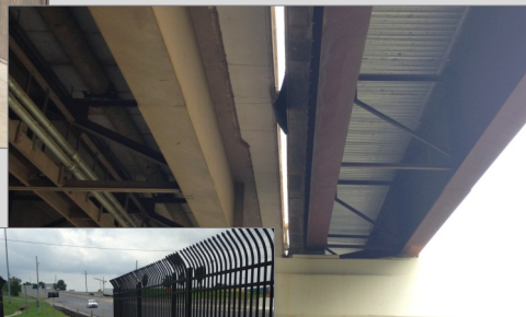
Shared Use Pathway added to existing Hwy 129 expressway bridge over the Tennessee River in Knoxville, TN. Top Image: Underside of structure; Bottom Image: Pathway view.
