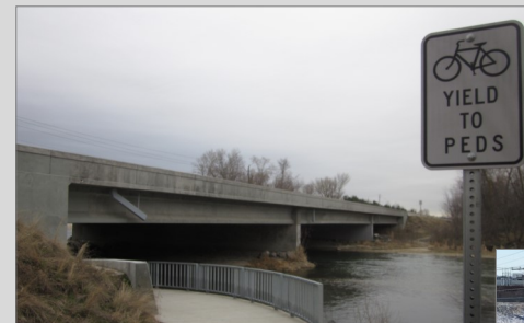
Shared Use Pathway retrofit under Highway 55 bridge over the Boise River in Eagle, ID.
