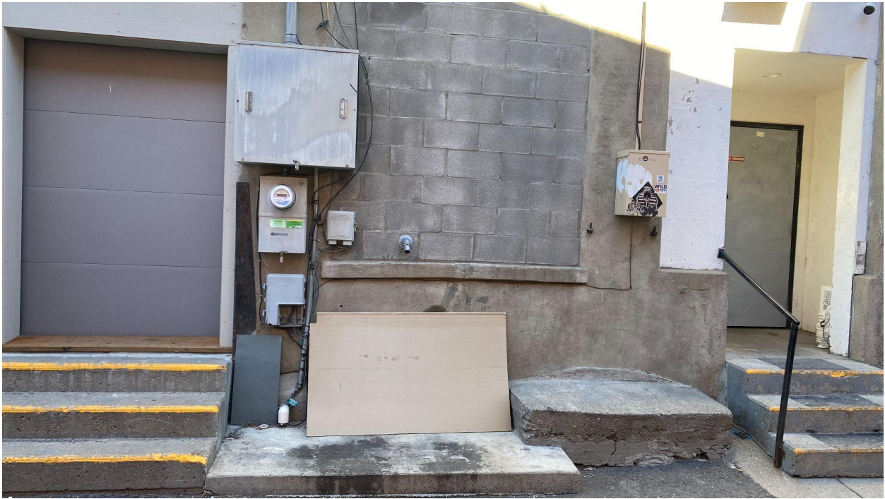
Rear Wall: Before and after remodel. Note: Security door has arrived and will soon be installed.
