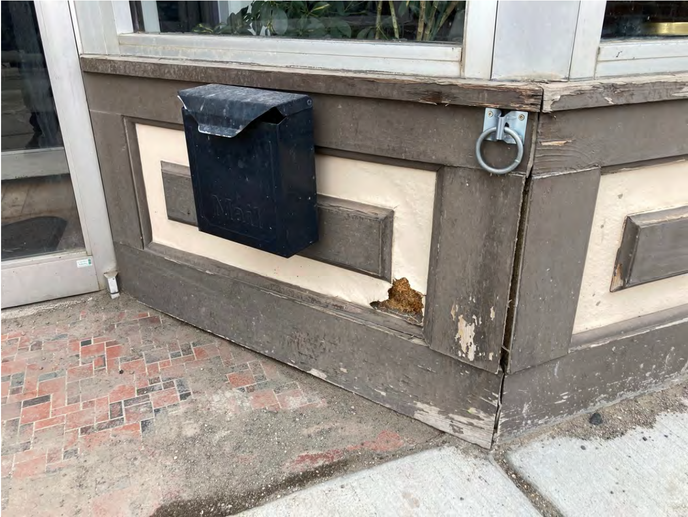
Deterioration of the façade as of March, 2022. No work has been done since that time. Please note the extensive repairs needed to woodwork elements and paint.
