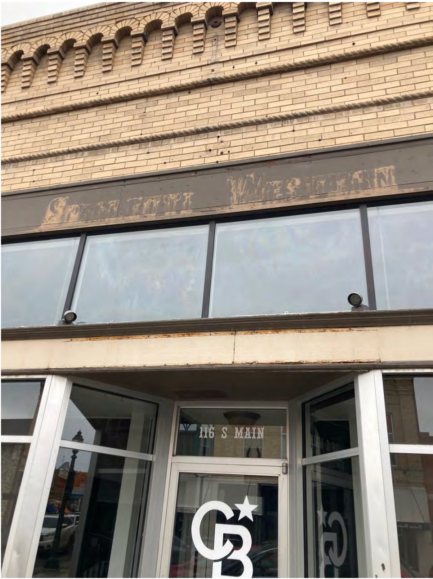
Deterioration of the façade
