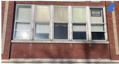
Lacking storm windows
