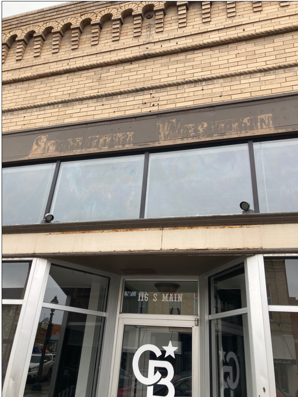
Deterioration of the façade
