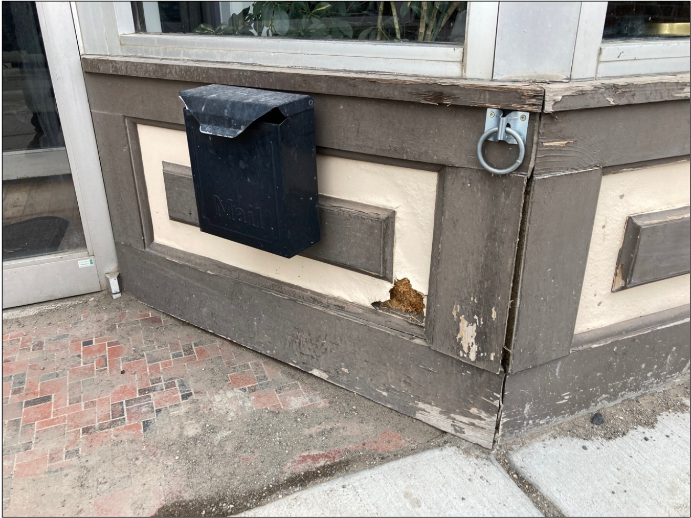
Deterioration of the façade as of March 2022. No work has been done since that time. Please note the extensive repairs needed to woodwork elements and paint.
