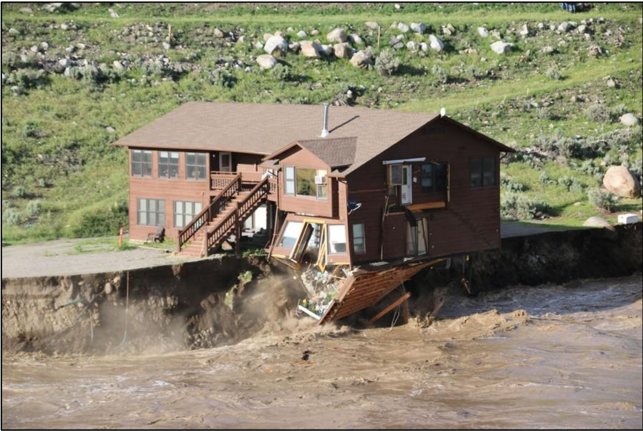
Figure 6. A National Park Service housing structure in Livingston, MT shown moments before falling into the Yellowstone River on June 13, 2022 (Gina Riquier / NPS).
