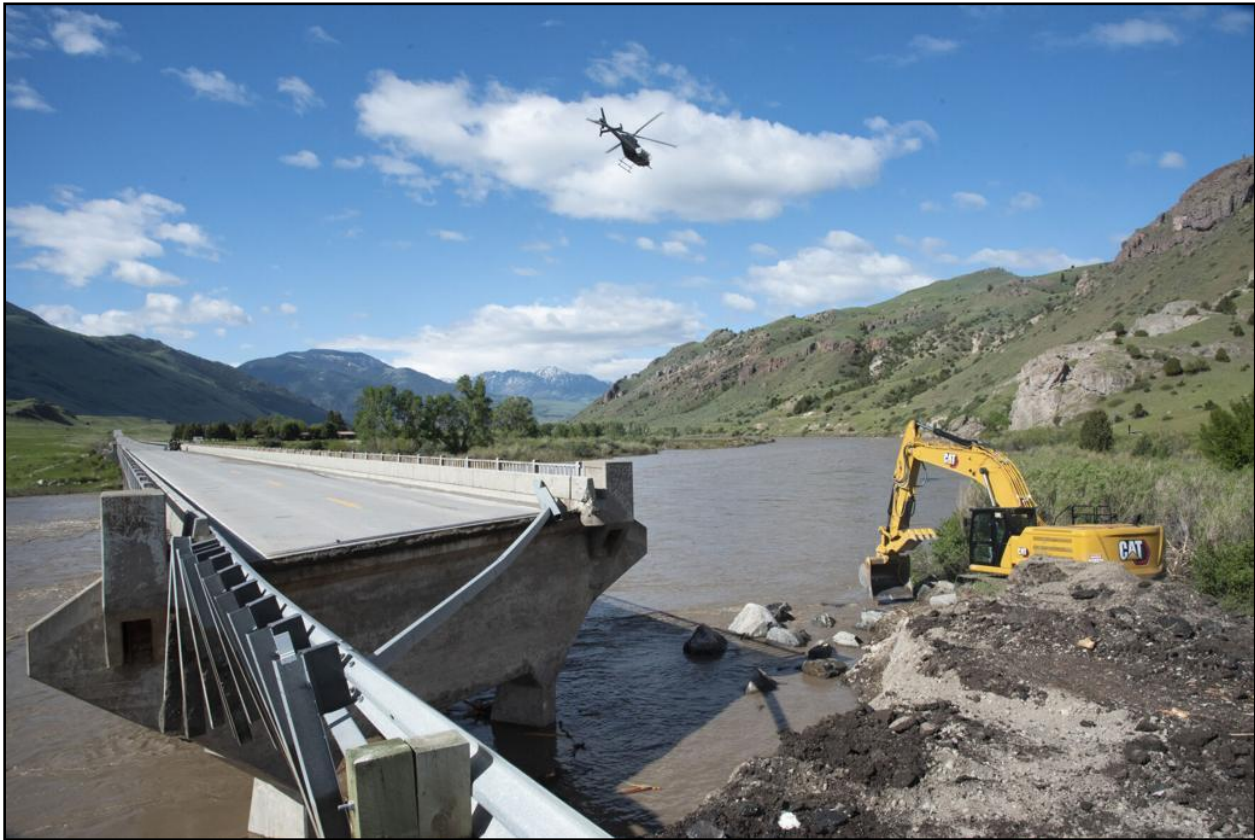
Figure 52. Point of Rocks Bridge showing where the northern approach was flanked during the flood. (Samuel Wilson/Chronicle/Report for America).
