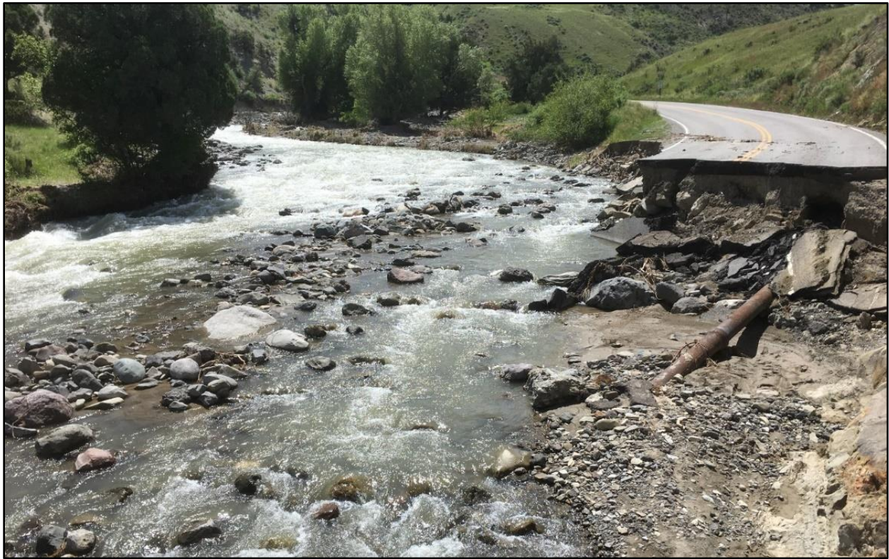
Figure 22. 2022 flood destruction of the Highway 89 North Entrance Road to Yellowstone National Park on the Gardner River, which joins the Yellowstone River at Gardiner.
