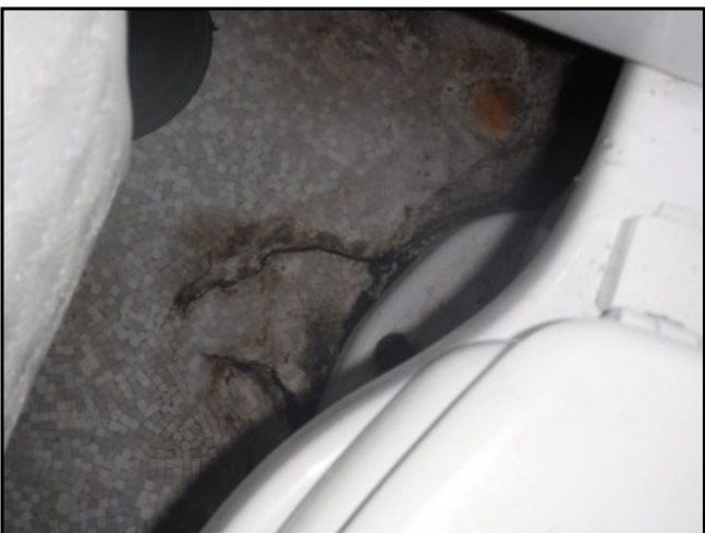
131 : Damage floor from leaking toilet
