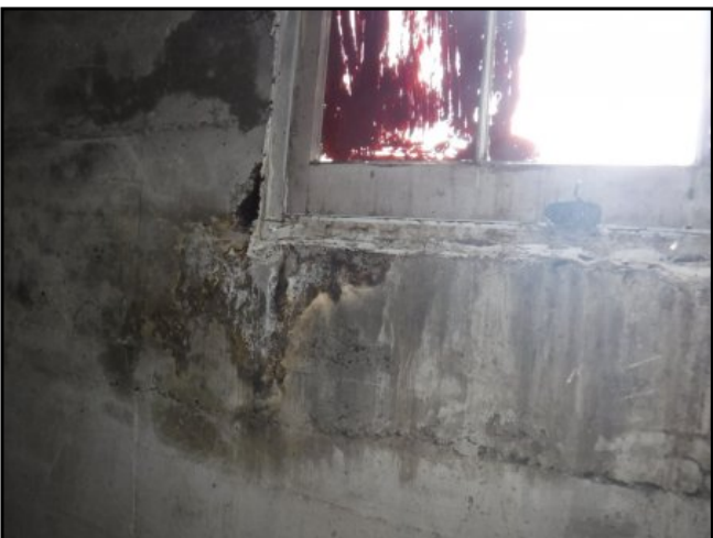
23 : Evidence of water intrusion at basement window
