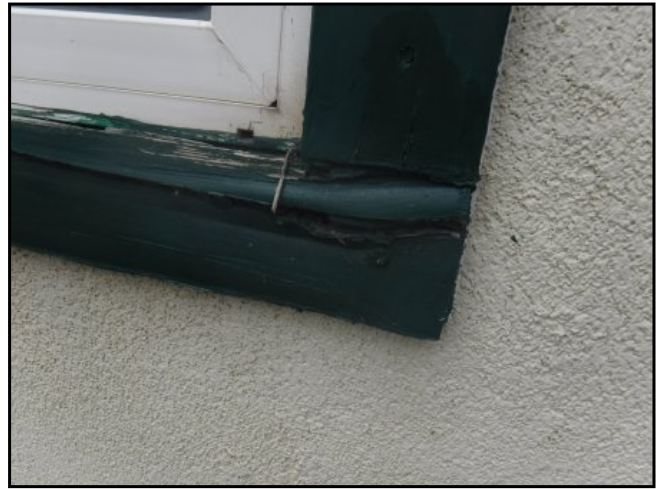
32 : Rot at window trim
