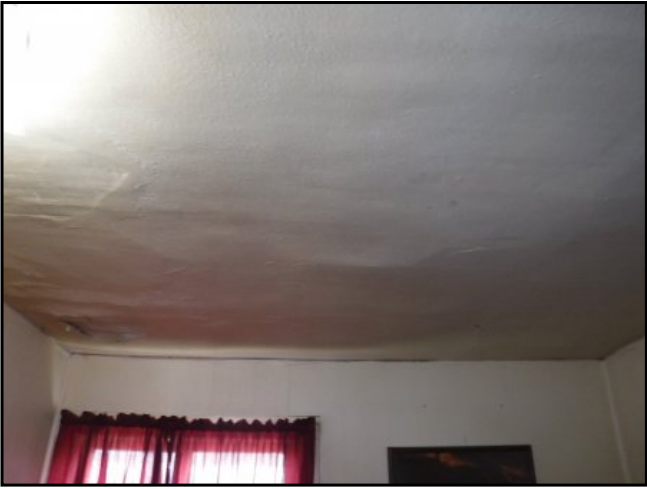
117 : Damaged plaster ceiling
