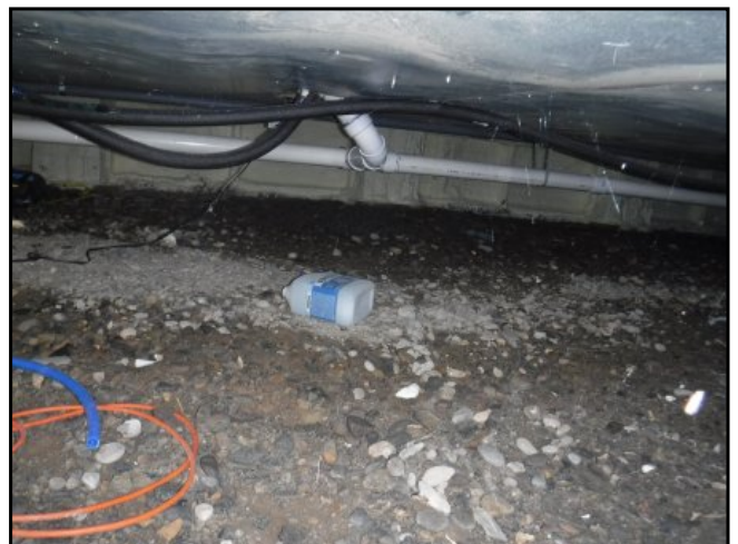
24 : View into crawlspace at the B Building showing cripple wall foundation construction
