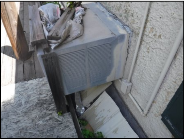
31 : Poorly installed AC unit sleeve
