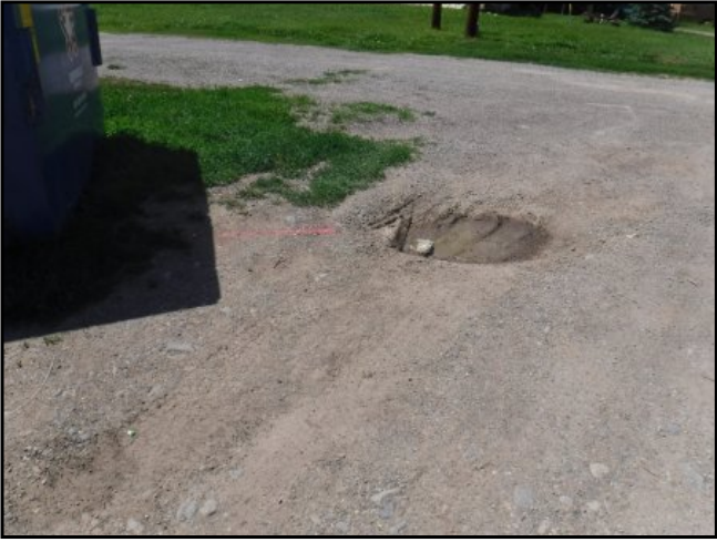
5 : Damaged road conditions in need of repair
