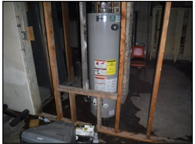
64 : Water heater for A1-2
