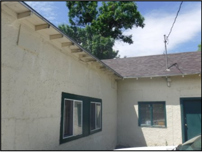
51 : Typical condition of stucco and roofing at the A building
