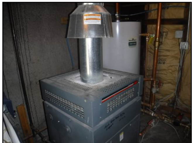
66 : Domestic water boiler and storage tank
