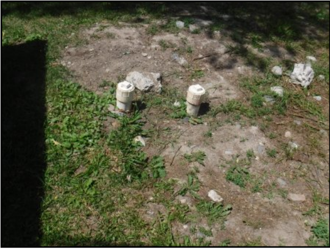
58 : PVC waste line clean outs
