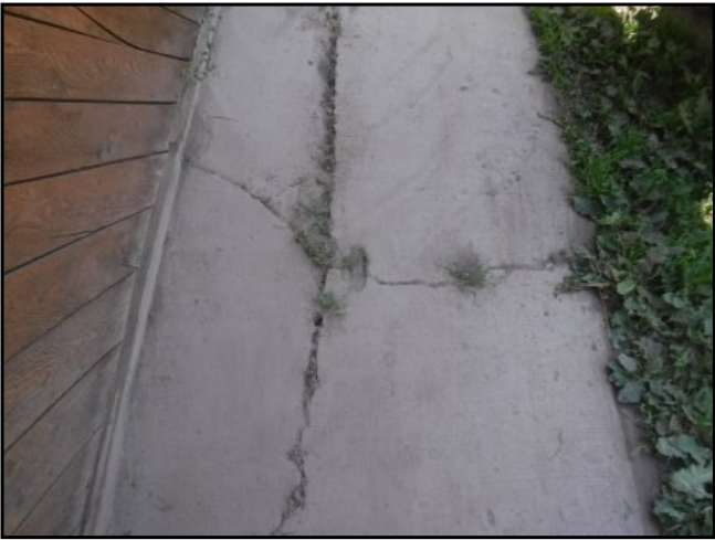
7 : Cracked and damaged pedestrian walkway at the C buildings
