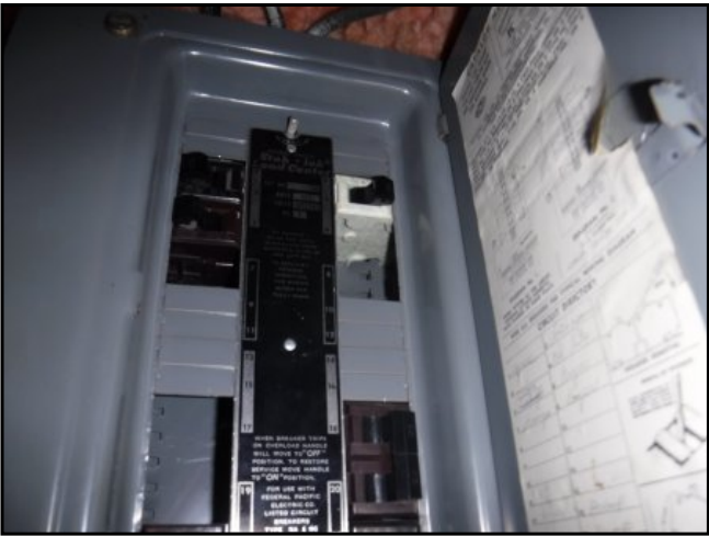
75 : Missing breaker covers at subpanel in basement of A1-2
