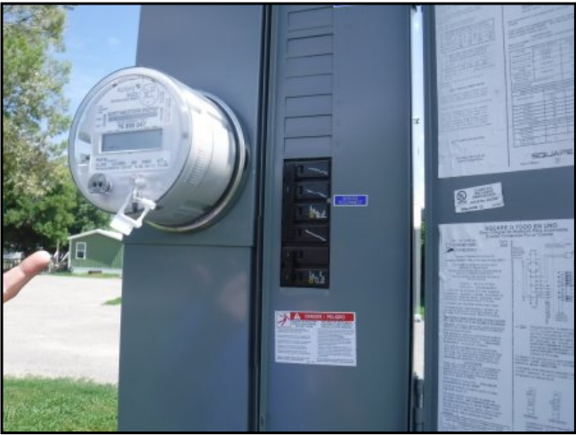
73 : 100 amp panel for the C buildings
