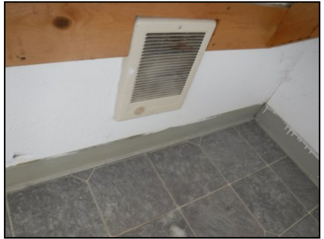
86 : Electrica wall heater at laundry room is non operational
