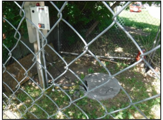
68 : Sanitary lift station
