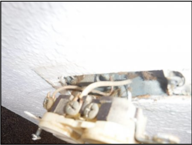
80 : Copper wiring observed in multiple locations
