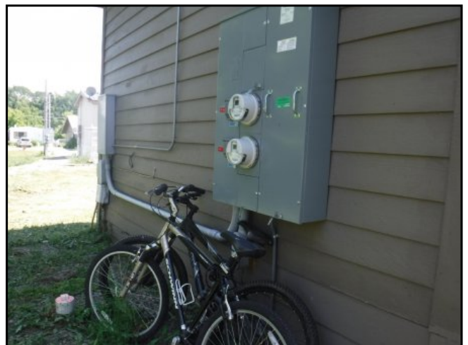
72 : Electrical meters for the B Building
