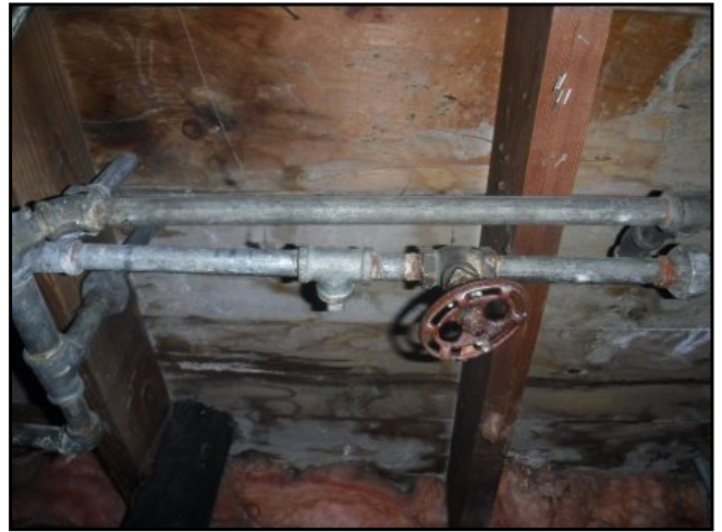
62 : Galvanized water lines
