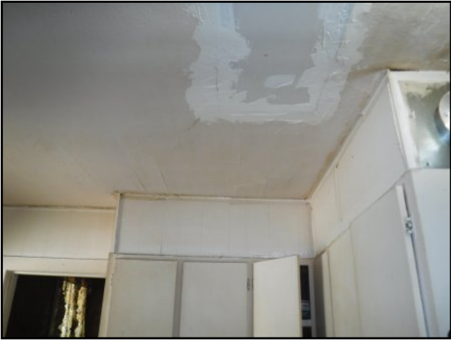
118 : Repaired ceiling fro previous roof leak
