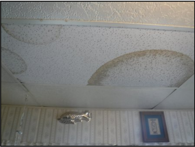
115 : Damaged ceiling tile from previous roof leaks
