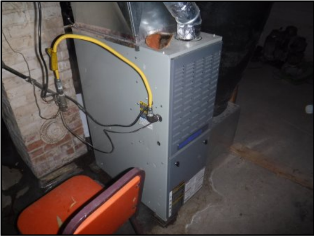
82 : Gas fired furnace for A2
