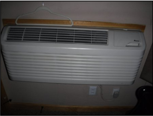
91 : Through wall heat pump for the B Building
