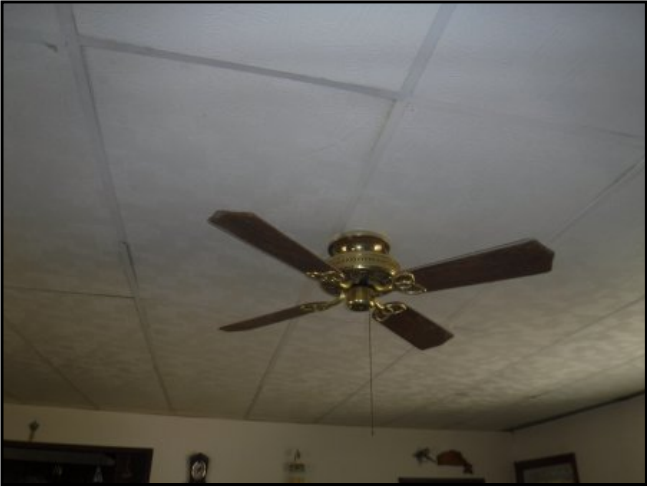
95 : Ceiling fan and dropped ceiling system
