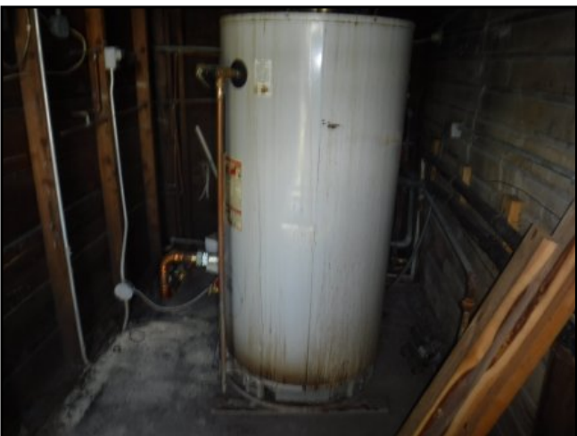
65 : 50 gallon water heater for units A1-2
