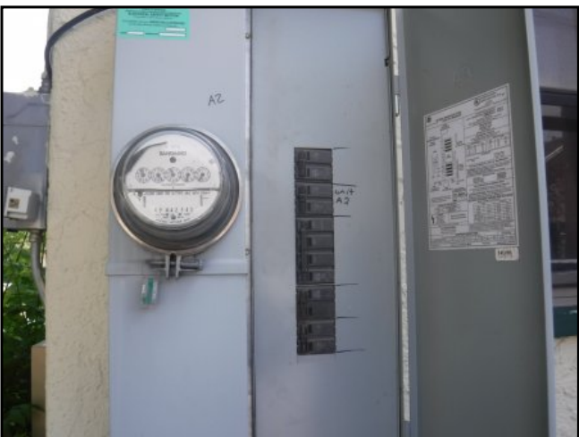
71 : Newer panel and meter for the A1-2 building
