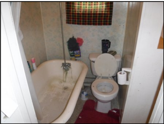
125 : Bathroom with older and worn plumbing fixtures
