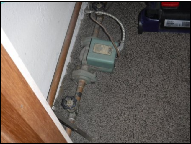
87 : Circulation pump for hydronic heating
