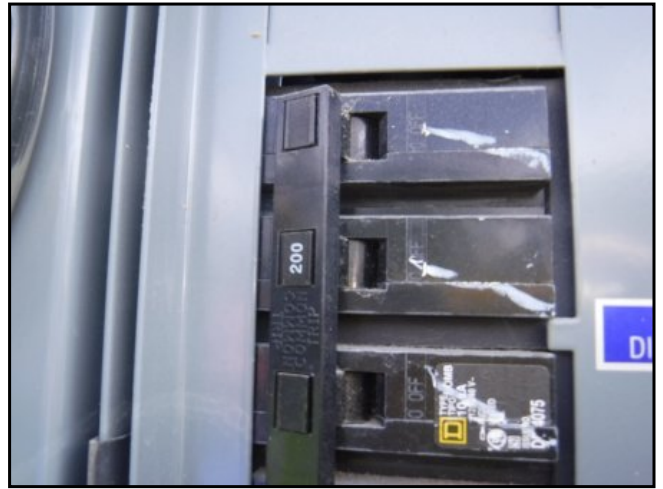
74 : 200 amp breaker for the A buildings
