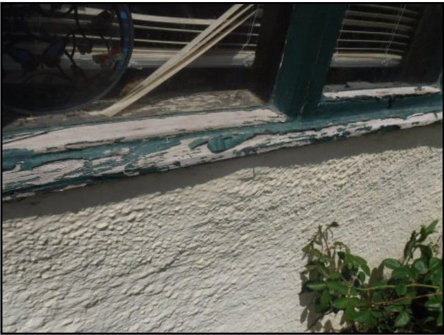
27 : Damaged trim and peeling paint
