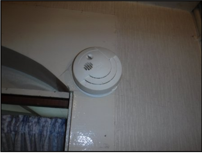
96 : Combination smoke and carbon monoxide detector
