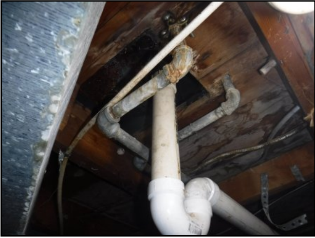
60 : Galvanized water lines and active water leak in basement of A1-2
