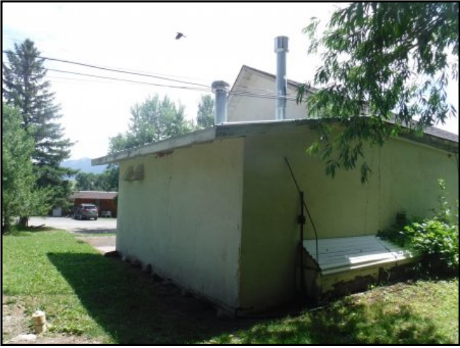
53 : Water heater enclosure
