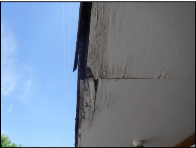
29 : Soffit damaged at the C buildings
