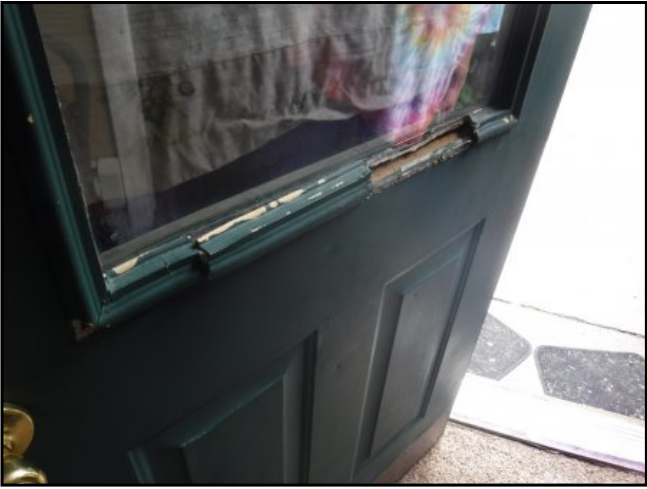
45 : Damaged door are unit entry
