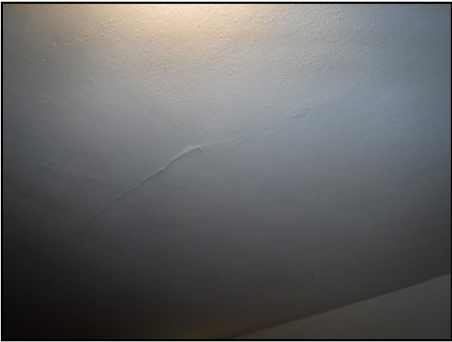
116 : Cracked plaster ceiling
