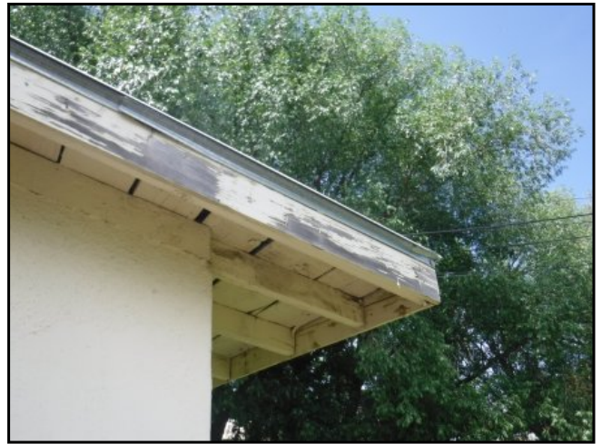
28 : Peeling paint and rotted fascia board
