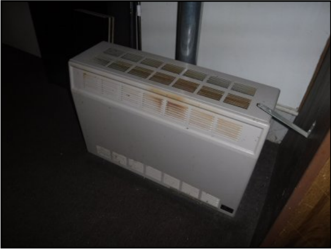
84 : Older space heater
