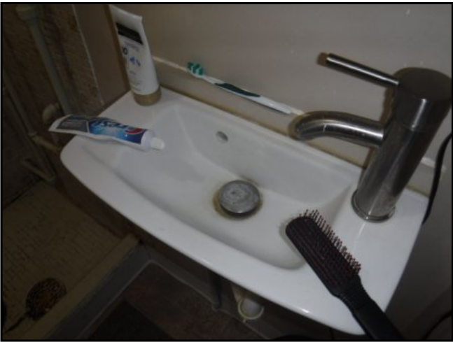
129 : Older wall mounted sink
