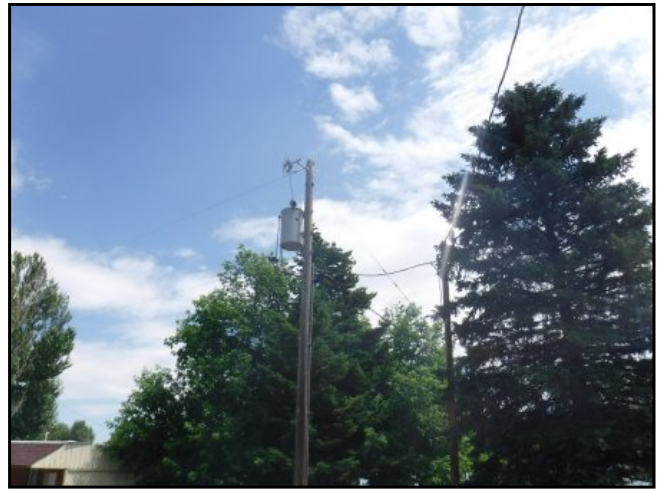
70 : Pole mounted electrical transformer
