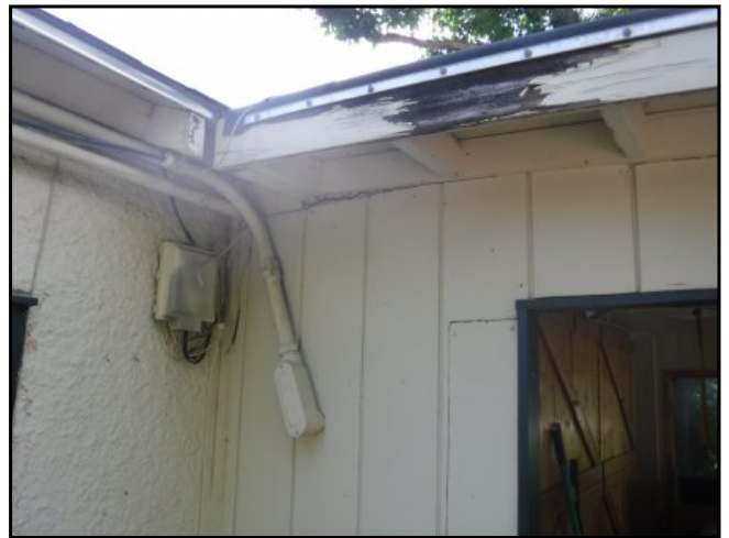
30 : Rotted fascia boards
