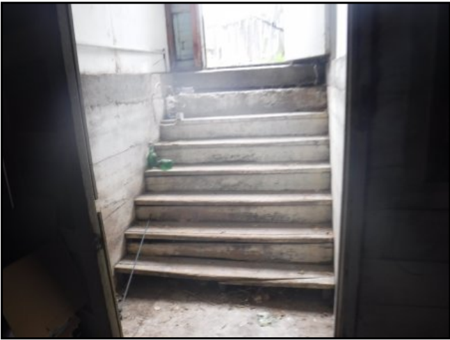
56 : Wood stairs leading to basement. Note lack of handrail
