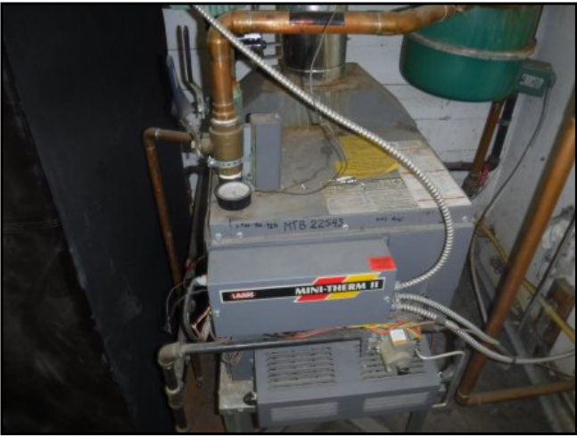
67 : One of two hydronic boilers for the Property
