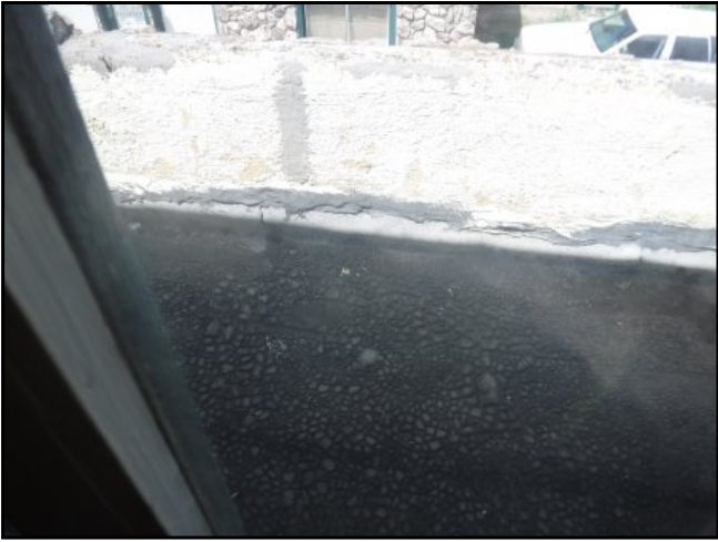
46 : Small balcony area at the A1-2 building
