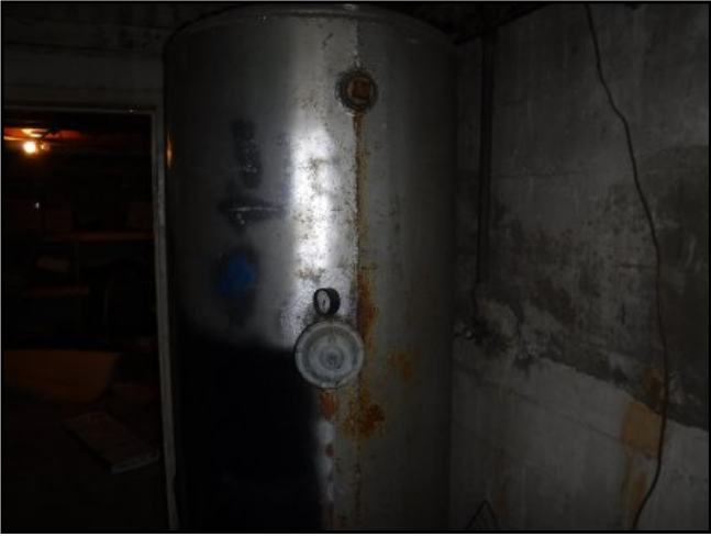
59 : Abandoned water storage tank in basement
