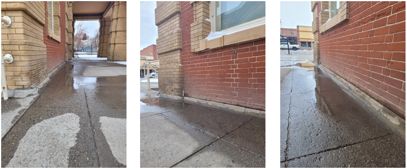
Figure 1: Standing Water and Brick Damage to the Livingston Depot Baggage Building. Cutting a trench drain A trench drain in the concrete between the baggage building (currently the Gourmet Cellar) will remove standing water from the base of the building and drain it to the parking lot entrance.
