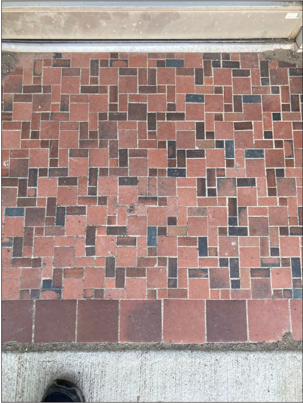
Existing tile entryway of our building This tile will be cleaned and restored if possible. If restoration is not possible, it will be replaced with matching or similar tilework.
