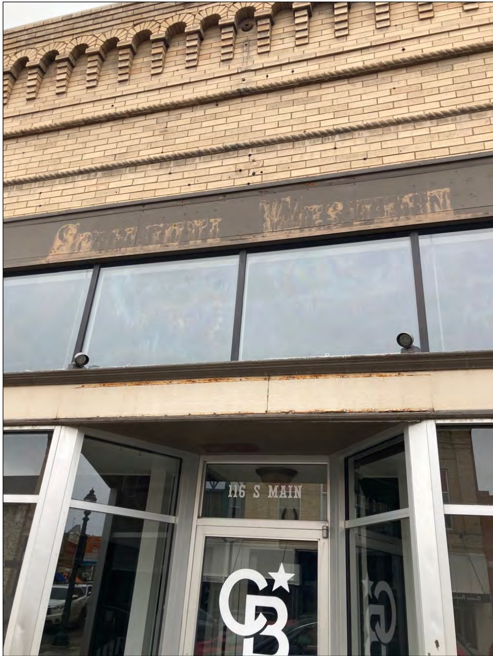
Deterioration of the façade
