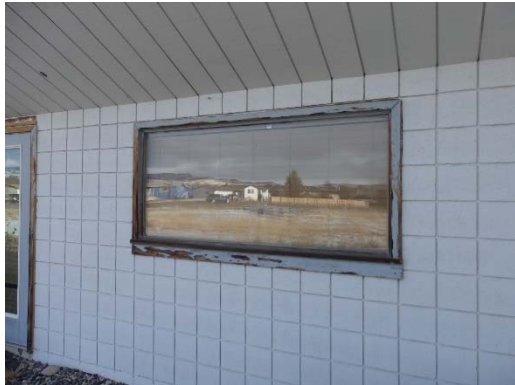
Deteriorating window casing.
