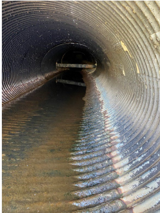
View of interior of pipe. Corrosion evident at interface of baseflow (water), air and steel pipe. An obstruction (gasline) is evident in this photograph.
