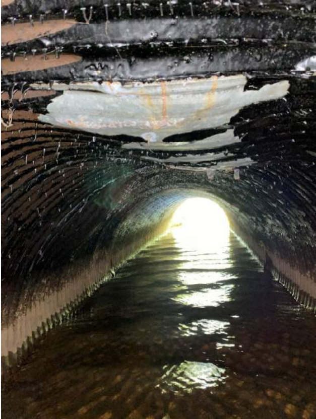
Picture 5: 6" bulge shown in picture 4.
