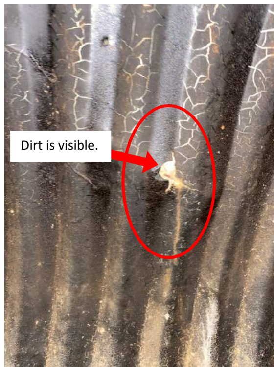
Picture 4: Small rupture close to upstream headwall. Small traces of dirt.
