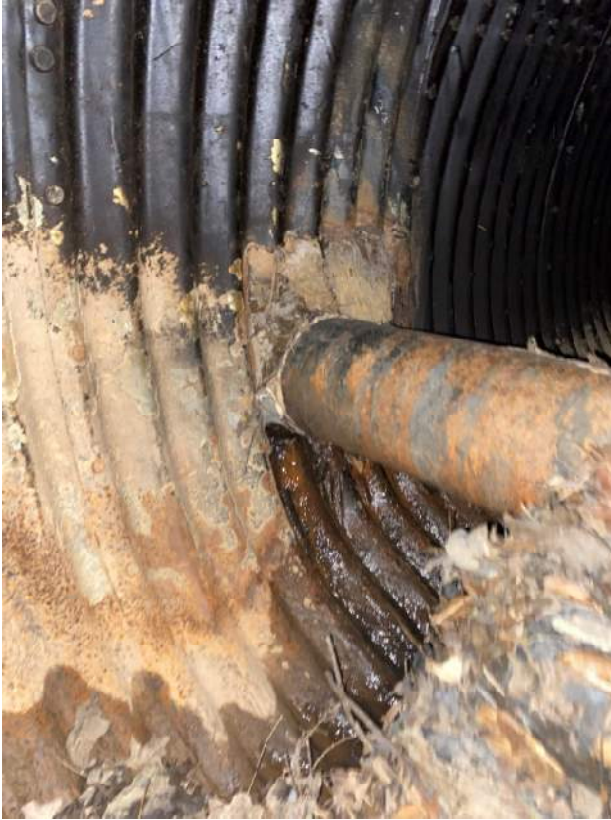
Picture 13: Small gap where pipe penetrates. Some sediment is escaping into the pipe.
