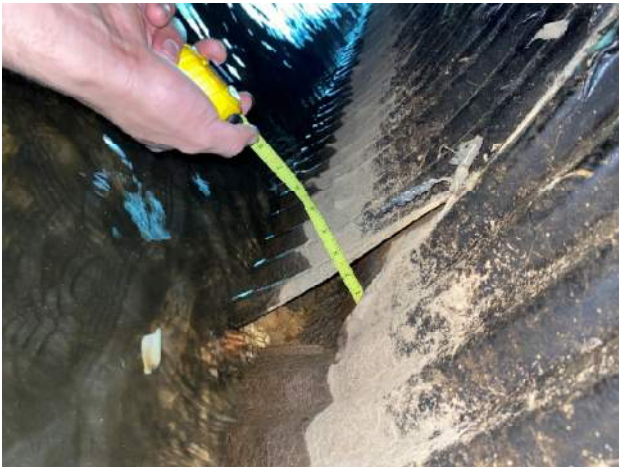
Picture 7: \pm 2 " gap at pipe joint.
