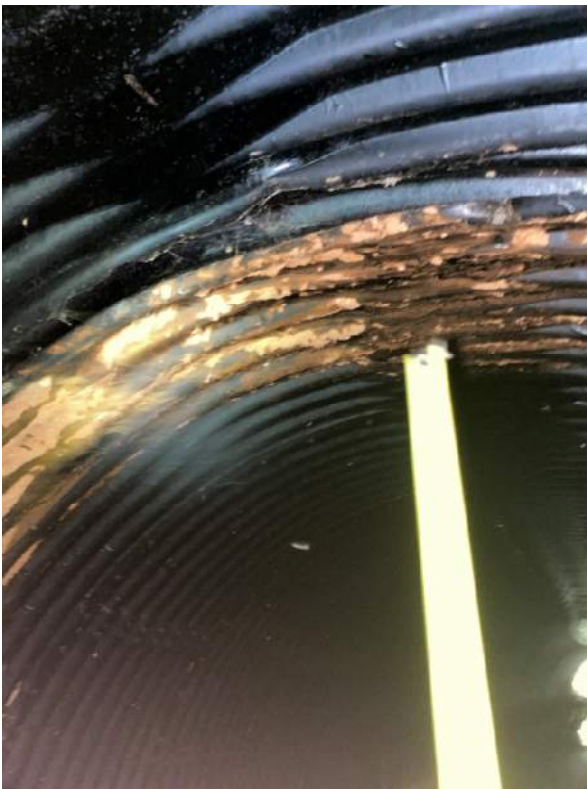
Picture 11: Corrosion on top of pipe.
