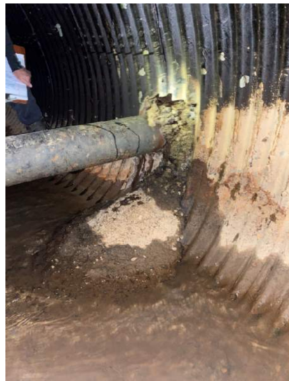
Picture 12: Water pipe crossing \pm 30' from upstream headwall. Penetration sealed with concrete. Spillage present.
