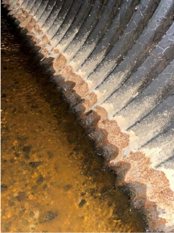
Picture 7: Corrosion along flowline but invert of pipe is solid.
