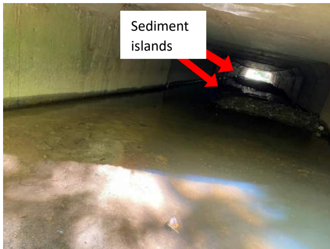
Picture 3: Left box culvert (facing East/downstream) has about 2' of sediment. There are islands of sediment about a quarter of distance downstream and halfway through the culvert causing 6" of ponding.
