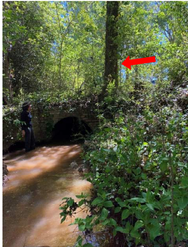
Picture 8: Downstream headwall. Large tree sits on top of headwall.
