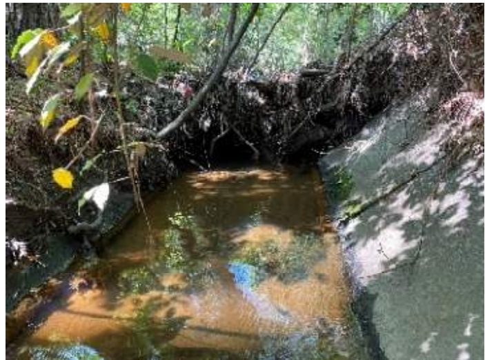
Picture 15: Logs and branches have clogged up the flume upstream of the pipe. Lack of freeboard endangers adjacent town homes.
