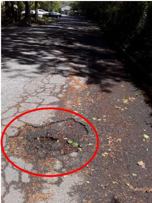
Picture 22: Second pothole on road in the vicinity of the pipe.
