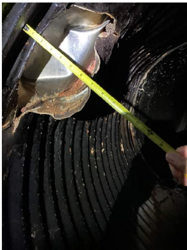
Picture 3: The pipe is damaged 10' from upstream headwall. 5" bulge and sediment noticeable.
