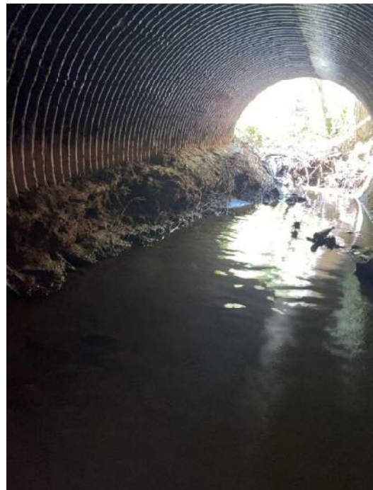
Picture 16: Solid sediment berm on the upstream end of the pipe.
