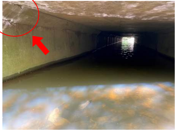
Picture 2: Right box culvert (facing East/downstream) has ~7" of sediment. Very small chips present in concrete at the south end in the top left corner (as seen in the picture).
