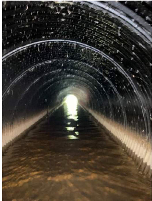
Picture 2: 6"-18" of sediment in pipe bottom.
