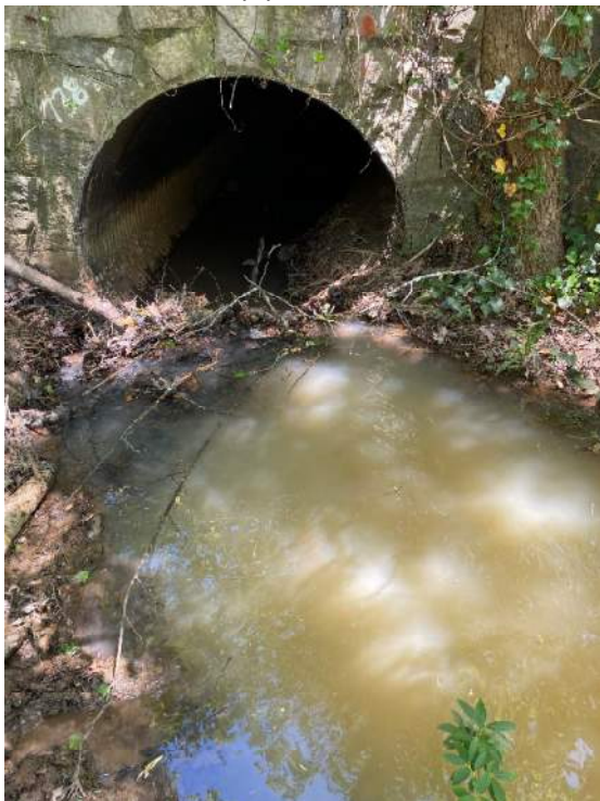
Picture 19: Water ponding up at upstream headwall.
