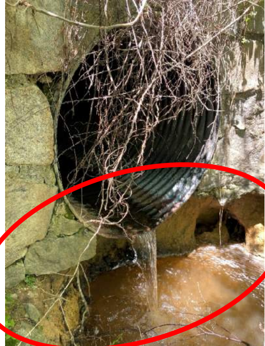
Picture 14: Undermining at downstream headwall. The grout at joints is loosening and falling out in headwall. Rip-rap recommended.
