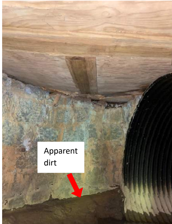
Picture 5: Customized junction box where pipe turns. A small embankment of dirt against one of the walls.
