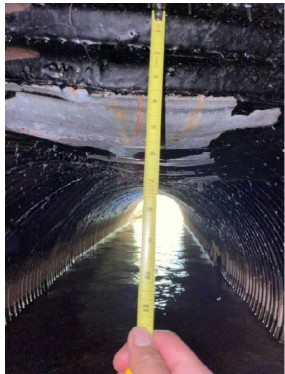
Picture 4: Approximately midway through the pipe a 6" bulge protrudes \pm 3' along the top of the pipe.
