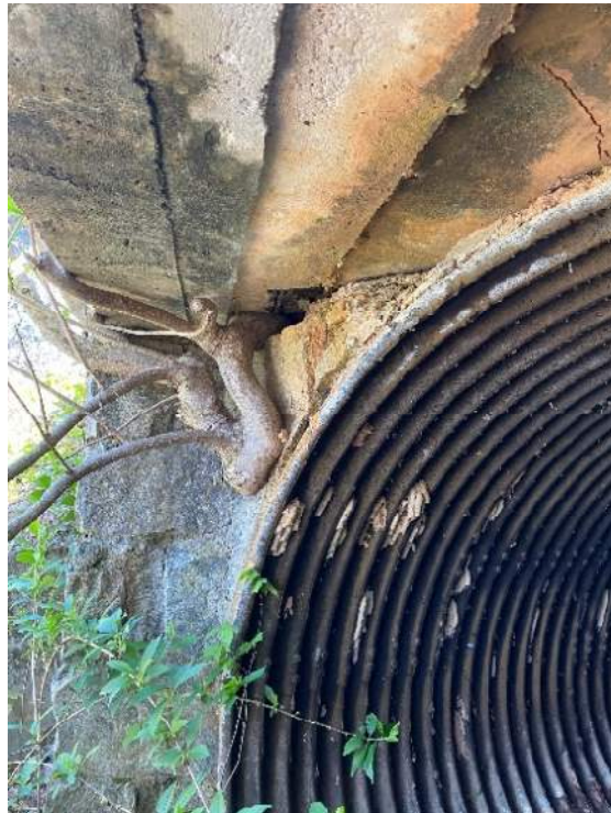
Picture 2: A tree is causing cracks in downstream headwall.
