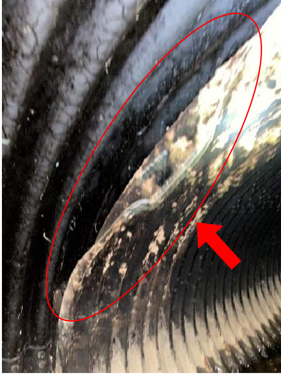
Picture 12: Bent pipe about 15' from upstream headwall.
