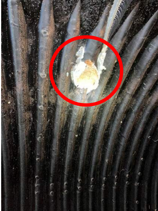
Picture 5: Small round rupture about 4" wide about 60 feet from downstream headwall. Possibly from repair work. No sediment visible.
