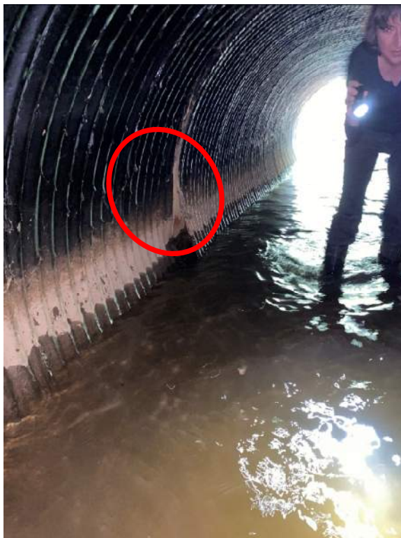
Picture 3: Gap at pipe joint.
