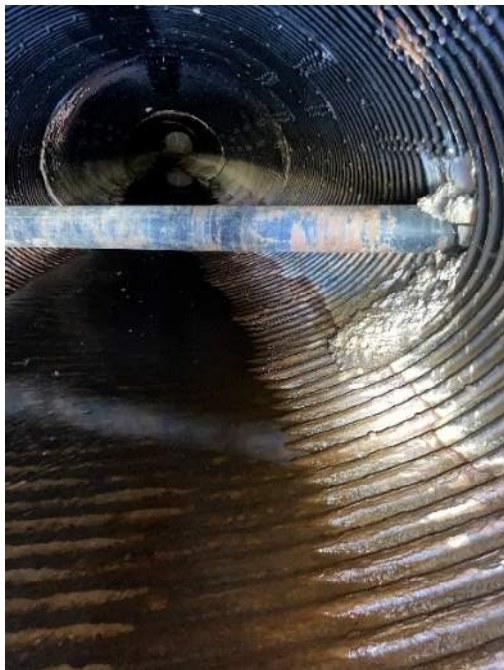
Picture 3: The invert of the pipe was somewhat corroded but solid. The crossing pipe \pm 25' from downstream headwall appears to be a water or sewer pipe. Penetrations appear to be sealed with concrete. Spillage present.
