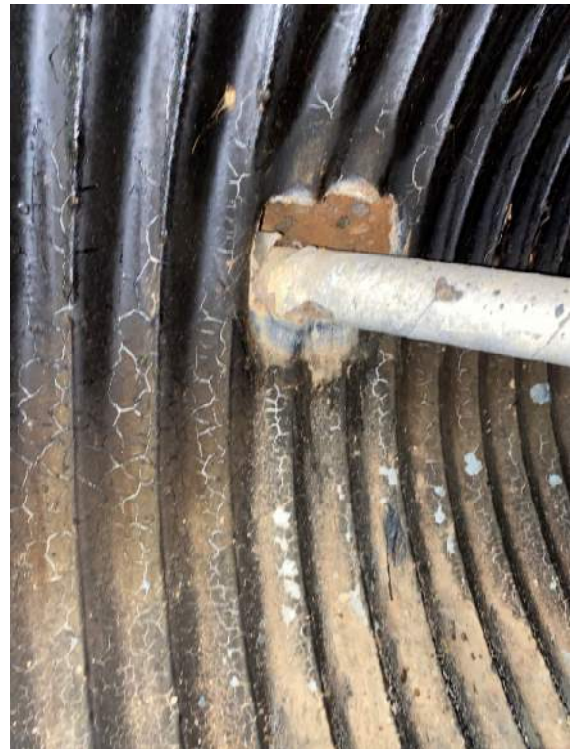
Picture 10: 4" pipe crossing close to downstream headwall. Dirt is visible where pipe penetrates.
