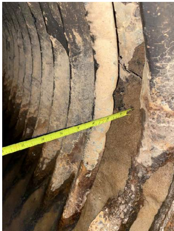
Picture 4: 2" gap between pipes at pipe joint. Some sediment making its way into the pipe.
