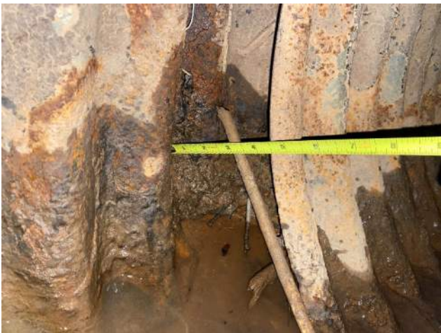
Picture 15: Gap shown on picture 14 at pipe joint. Some sediment is infiltrating.
