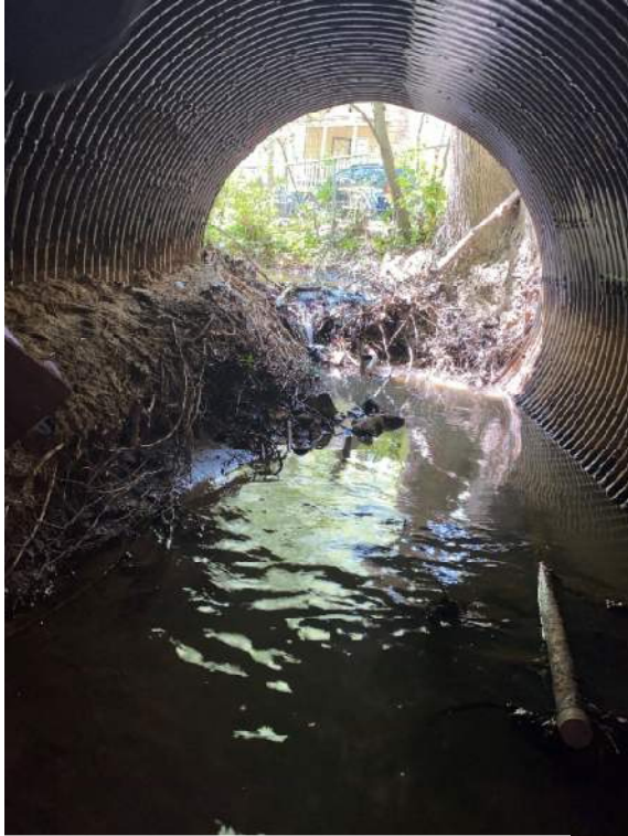
Picture 17: Branches, logs, and sediment clogging the upstream headwall of the pipe.
