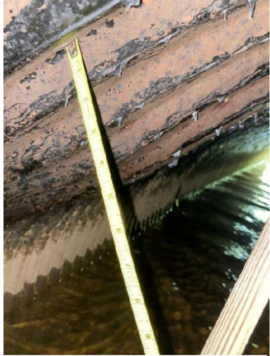
Picture 6: \pm 4 " bulge protrudes from the side of the pipe.
