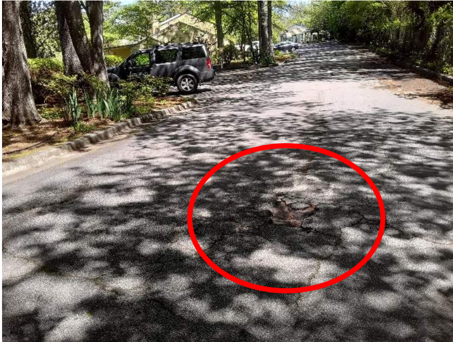
Picture 21: Pothole on road in the vicinity of the pipe.
