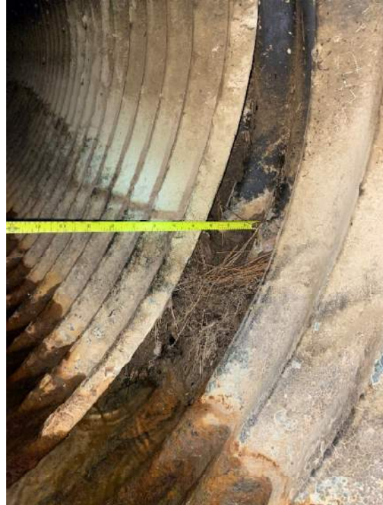
Picture 6: 3" gap at joint. Sediment present.
