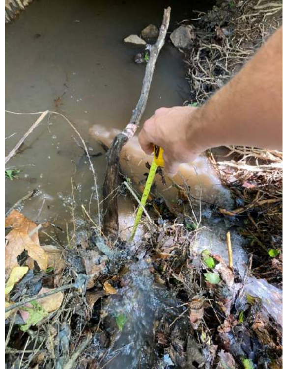
Picture 18: 1.5-2" of debris/sediment build up at upstream headwall.
