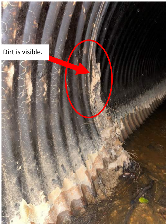
Picture 5: Gap at pipe joint \pm 20' from upstream headwall. Small traces of dirt.
