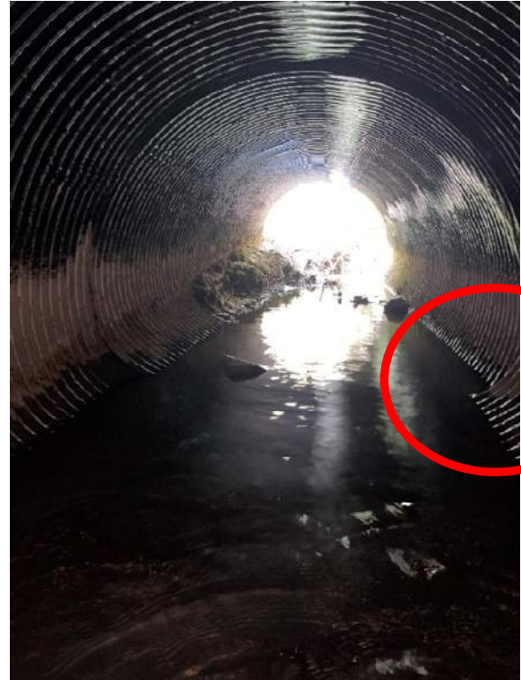
Picture 14: Gap between pipes at pipe joint. Gap located \pm 25' from upstream headwall.
