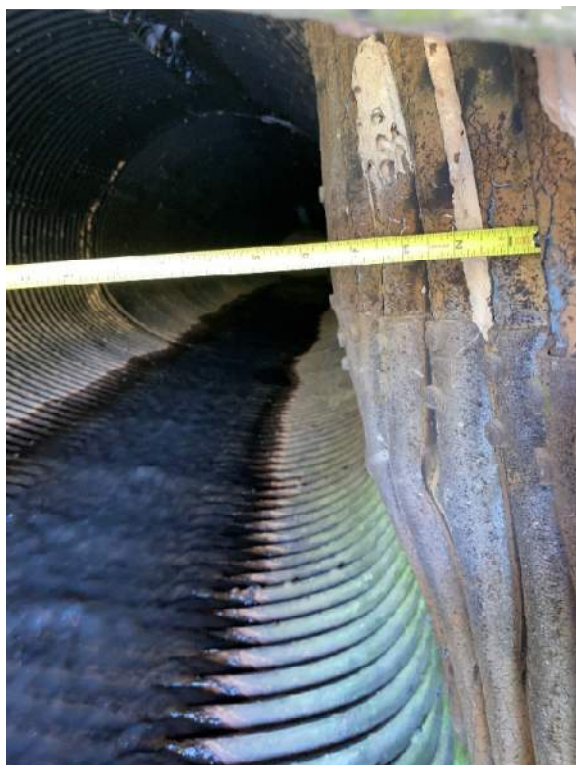
Picture 3: 5" bulge next to pipe in picture 2.
