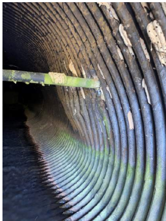
Picture 2: Gas pipe crosses at \pm 5' from downstream headwall.
