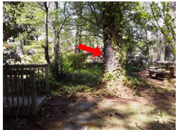
Picture 23: Tree appears to be above the pipe's path.
