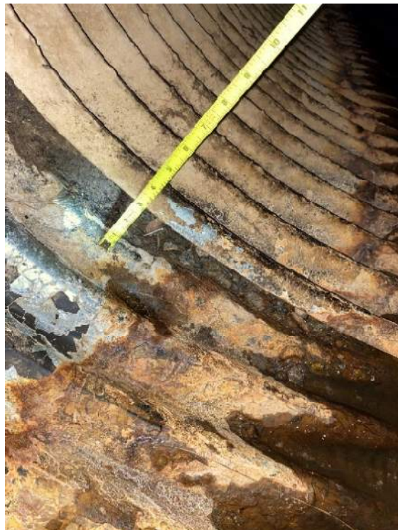
Picture 4: 3" gap at joint.
