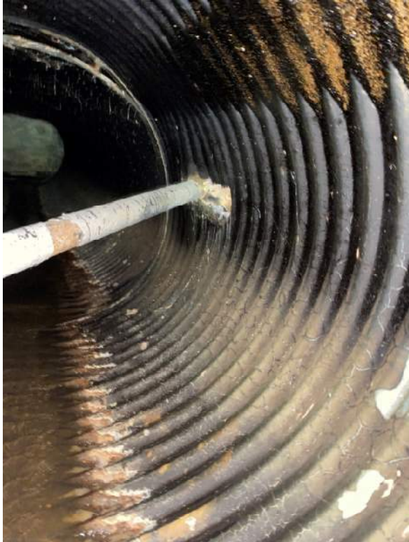
Picture 11: Other end of crossing pipe shown on picture 8. Dirt visible where pipe penetrates.
