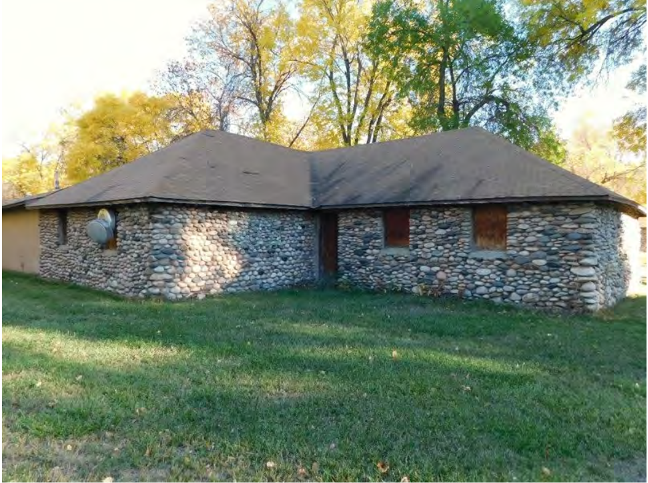
MT_YellowstoneCounty_RiversidePark_0018. Rifle Club building, view looking southeast. Northwest corner of the long building. October 07, 2023.
