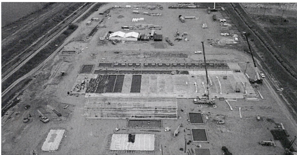
Source: Galvan Decl., Ex. 13 (Photo of NorthWestern Energy Laurel gas plant construction (Nov. 8, 2022))
