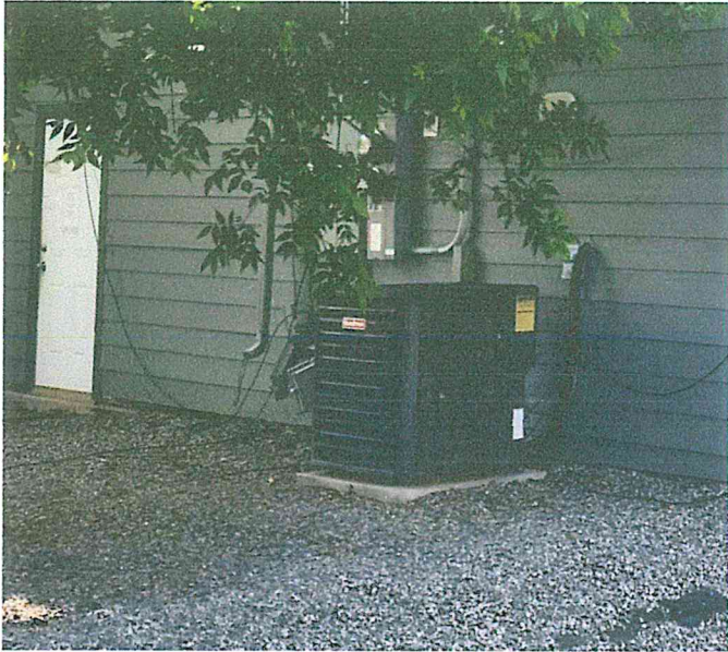
201 E. Main Street- HVAC -Old Unit
